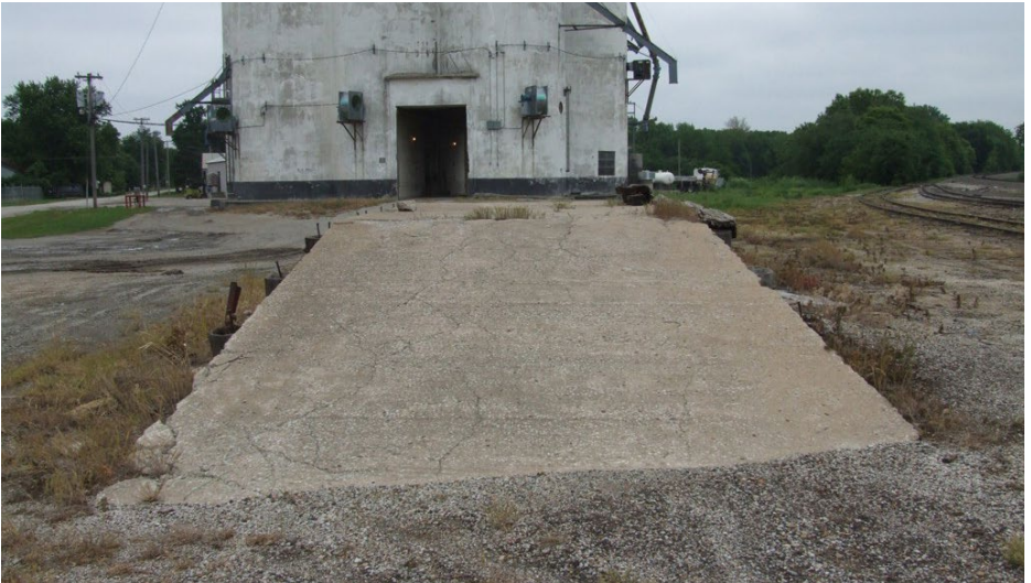
4. The ramp end of the loading dock, looking north. The interior of the entire structure was filled with sand and a concrete liner applied on top of the sand. May, 2008. Photo by Jared Harper
