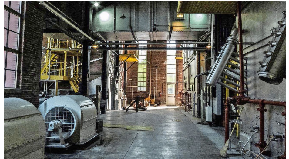
2. Inside the boiler house today. Boilers 16 & 17 are on the left, and Boiler 18 on right. The tube in front of No. 18 delivered coal to a crusher which fed fuel into the boiler's firebox. The building is a lot cleaner than when it was in operation with the coal-fired boilers. Philip Griffith photo
