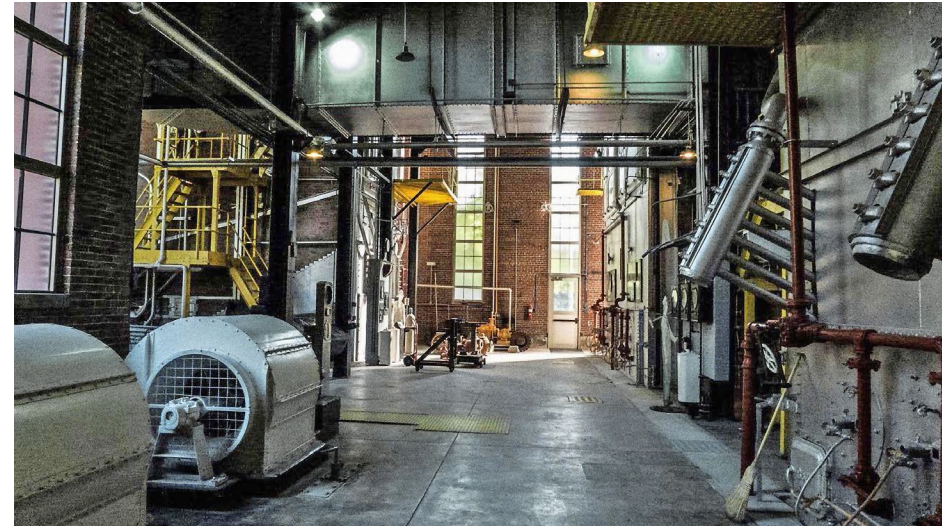
2. Inside the boiler house today. Boilers 16 & 17 are on the left, and Boiler 18 on right. The tube in front of No. 18 delivered coal to a crusher which fed fuel into the boiler's firebox. The building is a lot cleaner than when it was in operation with the coal-fired boilers. Philip Griffith photo
