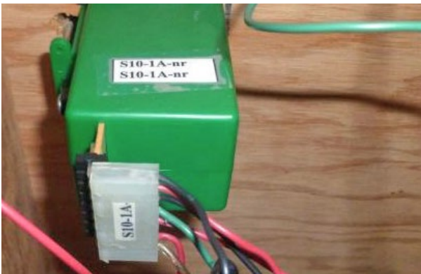
27. Identification labels have been applied to the switch machines and plugs.
