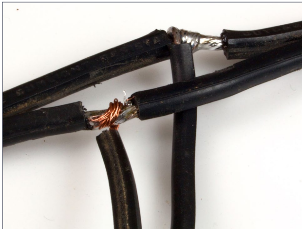
12. Connection between drop wires and bus wire. Two joints are shown in the photo. In the upper right is a completely soldered one – note the bright and smooth surface, indicating that enough heat has
