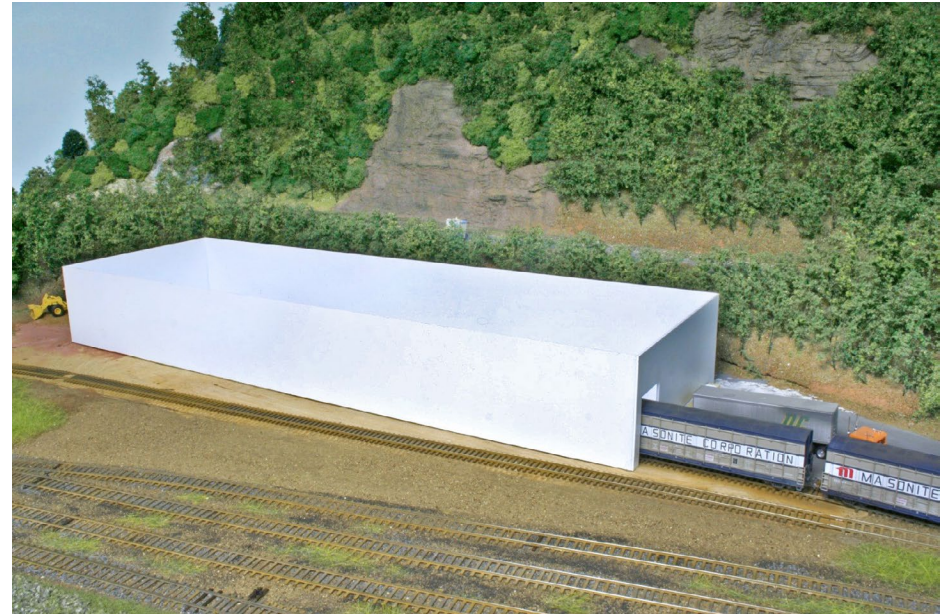
5. Here's the basic box of the structure in place, with a cut of cars to test the clearances.
