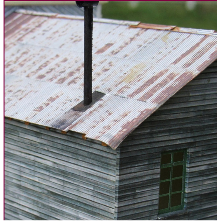
6. Distressed roof and ridge covering.
