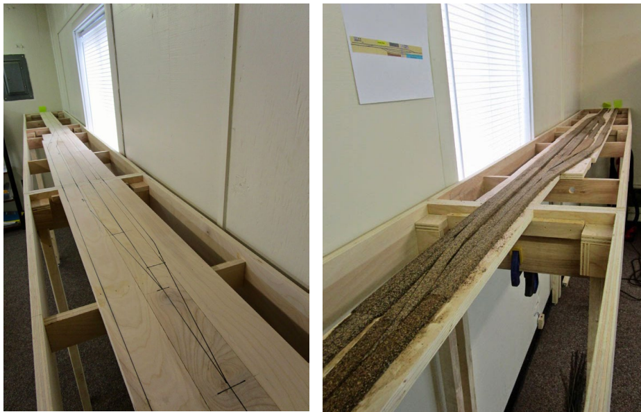
8-9. Laying out the track centerlines on the plywood, and then gluing down the cork roadbed.
