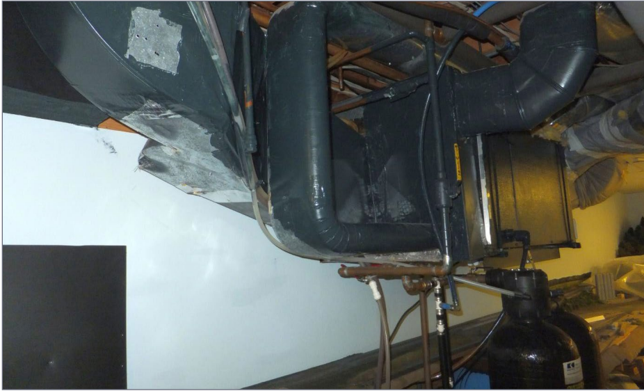
2. The air handler, water filters and associated piping. What's not to like?
