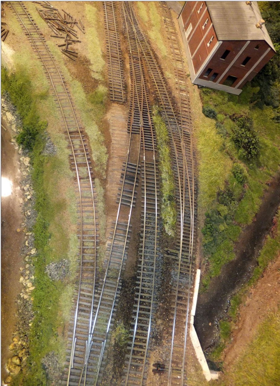
52. The area is now cleaned up and is ready for new track.
