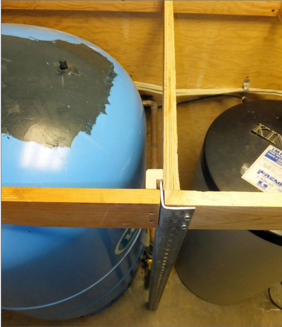
15. The pre-punched metal angle iron (one on each side of the Welltrol cylinder) proved to be a perfect small footprint support leg for the new bench work. I made a custom mounting bracket out of wood for the removable front piece. The bracket wrapped around each metal support leg on the left and right of the cylinder.
