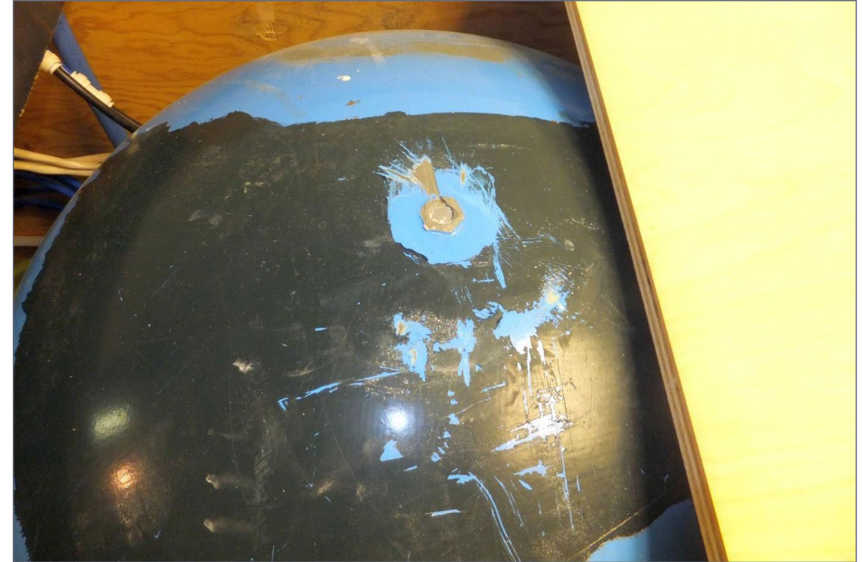
16. My friend Dave was alarmed when I took a Sawzall to the top of the Welltrol! I called the company on the phone to ask about this nut. It's used in the manufacturing process to allow them to transport the tank during construction and painting. Ask before you saw!
