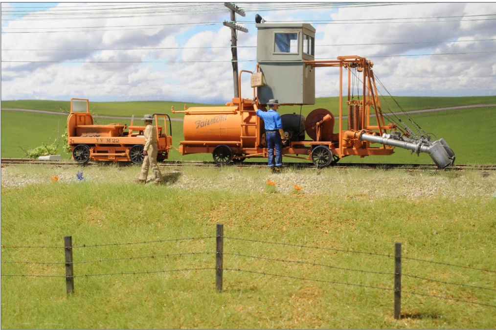
23. The gang car and weed burner. One of the weed burner operators is looking for a problem with it, giving the rest of the crew a short break.
