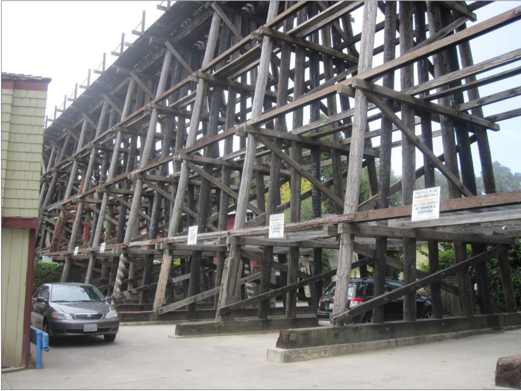
3. This old creosoted-timber trestle at Capitola CA has weathered to a silvery gray, but notice the brownish horizontal stringers, and the faded warning strips on the base level to the left. Dave Branum photo
