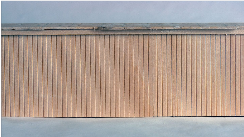
12. Showing where the door will go: I was not able to show all the steps in one photo, so there are three.
