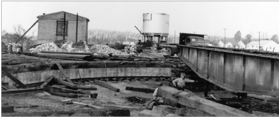
5. This photo was taken as the YV Merced yards were being scrapped, but it provides a fairly good view of the side of the oil house that faced the turntable in the foreground.
