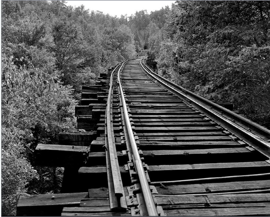
27. Twin Seam Mining Company - 5th Daniel Creek Trestle. View west from end of tunnel 3 across the fifth trestle up Daniel Creek. East end of tunnel 2 is in the distance. This trestle is about 350 feet in length. Note guard rails are on the outside of the running rails. William G. Gordon photo
