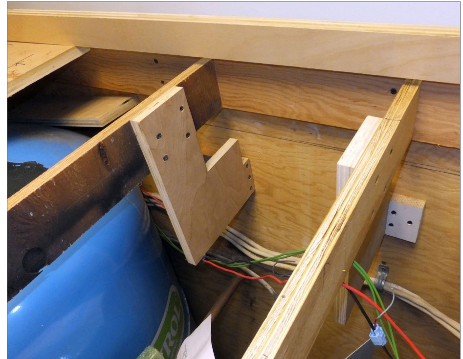
8. The pesky blue water pressure tank that has plagued many of my layout efforts was at it again! There was only one way to get two tracks to pass underneath Tunkhannock, and that was to sneak them behind the tank near the top. Clearances were tight – I just made it. The strange L-shaped plywood brackets were created so that I could chop off the existing joist ends. This was the area the new tracks needed to pass through.
