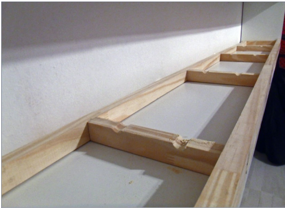
8. Building module benchwork using 1x3s and 1x4s, with some indents in the joists to allow running the wiring.
