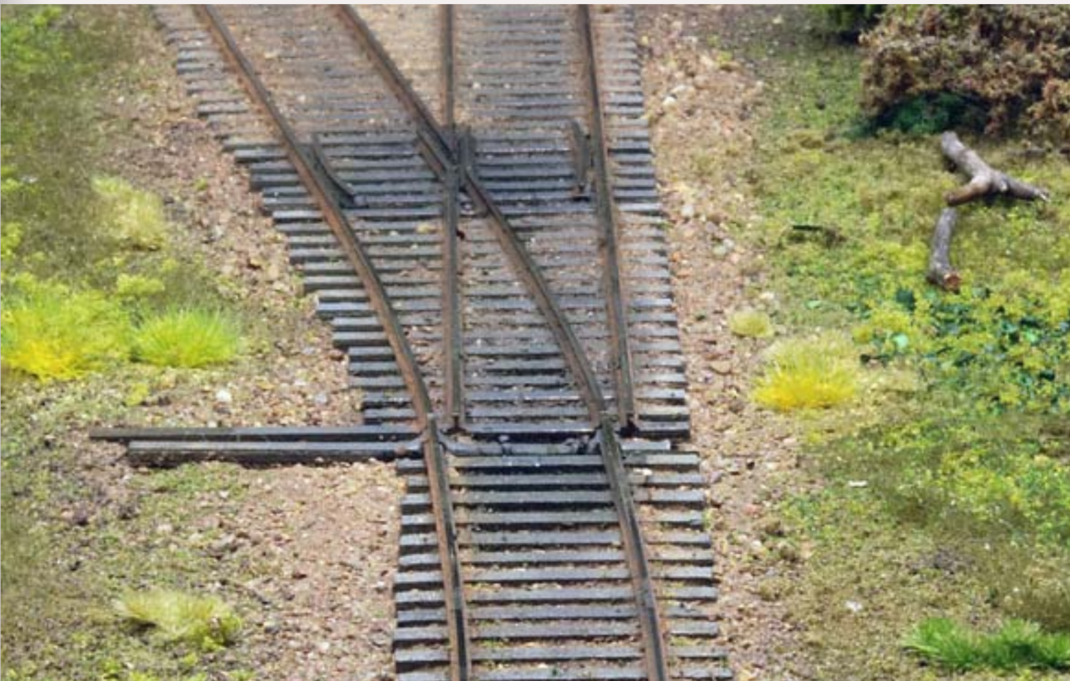
FIGURE 5: The bridge portion of a stub switch acts as a spiral easement into the curve of the diverging route by providing a larger radius at the start of the arc, and spirally getting sharper as it enters the frog of the switch.
