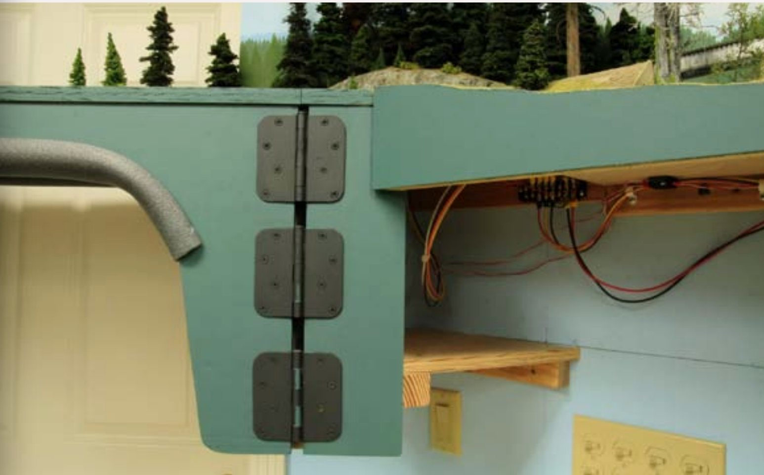
FIGURE 18: A movable bridge with track on it requires secure abutments. I used 'box' style construction to build mine. Note the three hinges. They need to be good quality because they set the horizontal alignment at the hinge end. If they get sloppy the tracks won't line up right. The axis the gate pivots on should be absolutely vertical.
