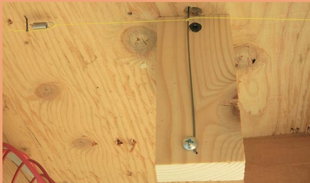
Figure 43: Switch points pulled by knob and shaft.
