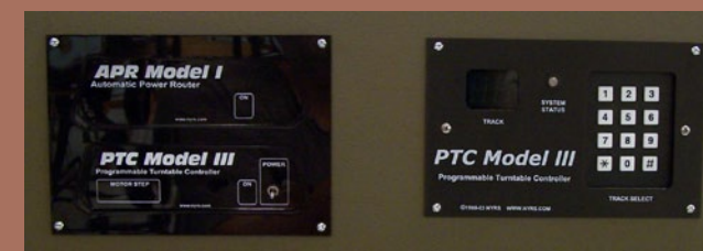
Figure 91: Fascia mounted components.
