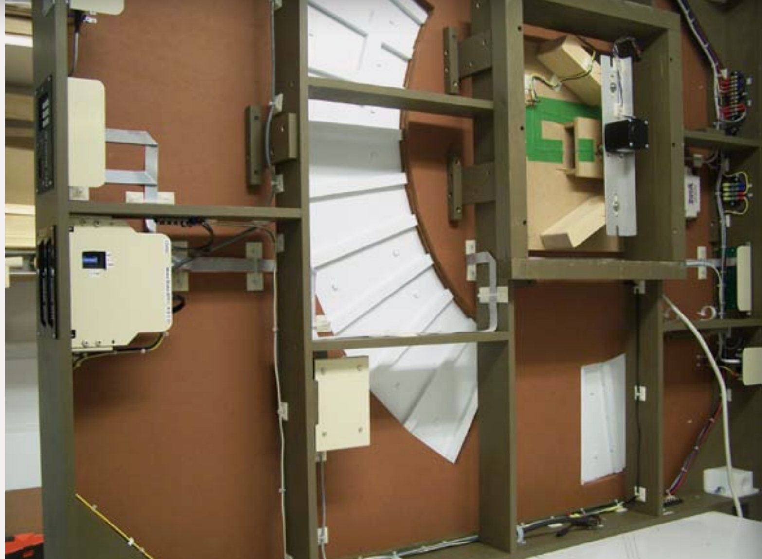
Figure 1: As we start into Part 2, we'll install the control wiring, the track, the feeders and program the NYRS system.
