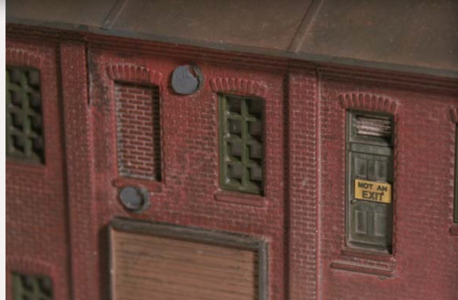
FIGURE 3: Splice on brick structure coincides with pilasters. The splice is just to the left of the loading door.
