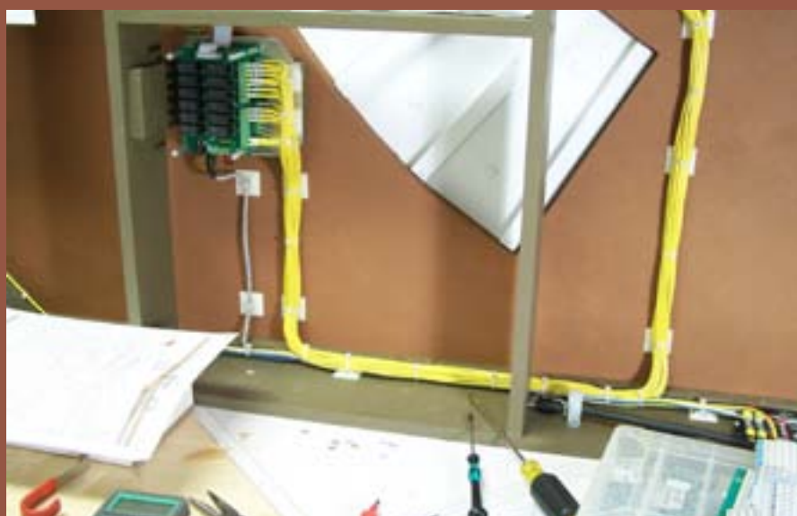
Figure 88: There are 21 wires coming in to the APR from each track. I used 18 gauge wire and made a neat bundle, identifying each on both ends. This is where proper documentation and neatness count should I need to troubleshoot later.
