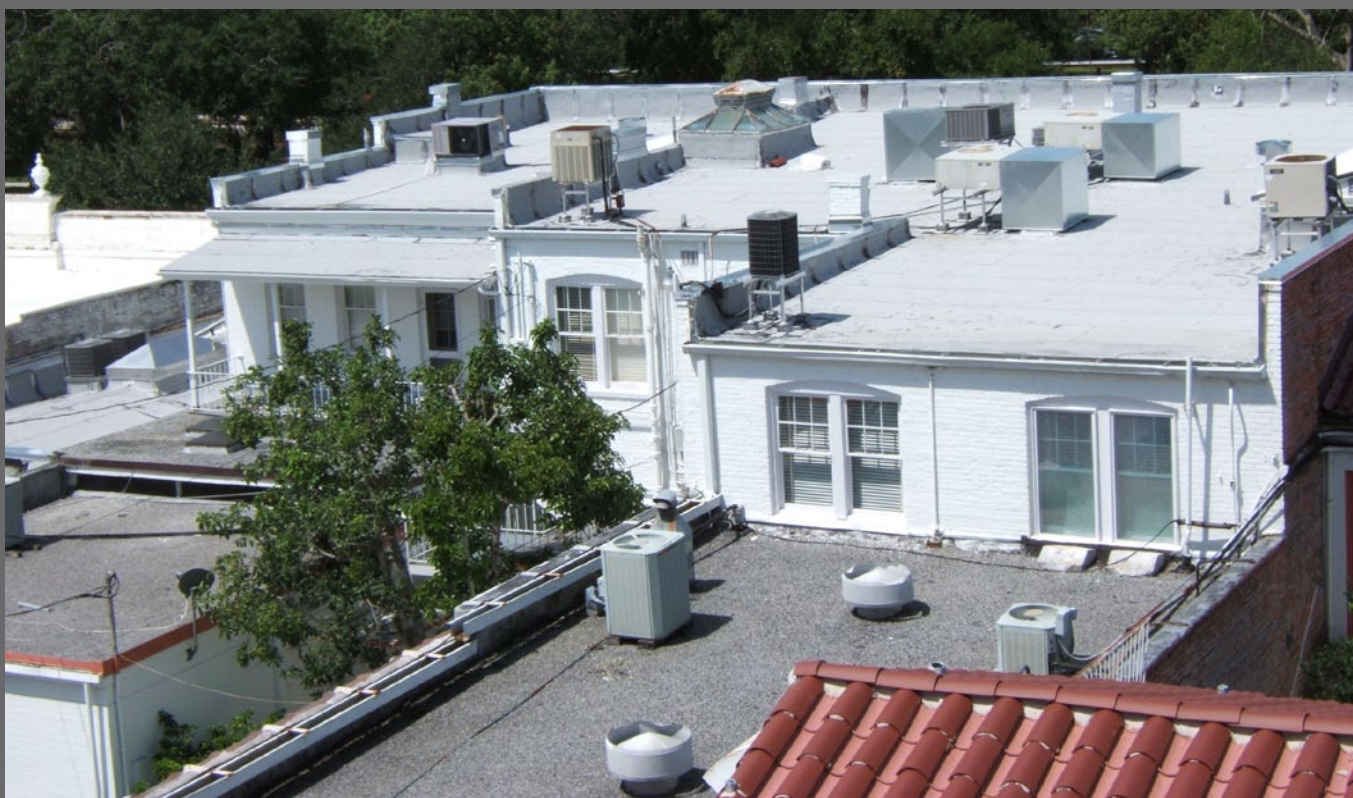
(Figures 58, 59, 60) These pictures show some prototypical roof tops in a block of stores that were built in the 1920s. Some of the roofs layouts are original and some have been modified.
