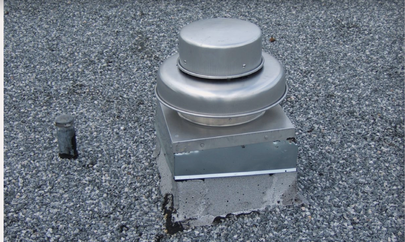
Figure 21: Restroom exhaust fan.
