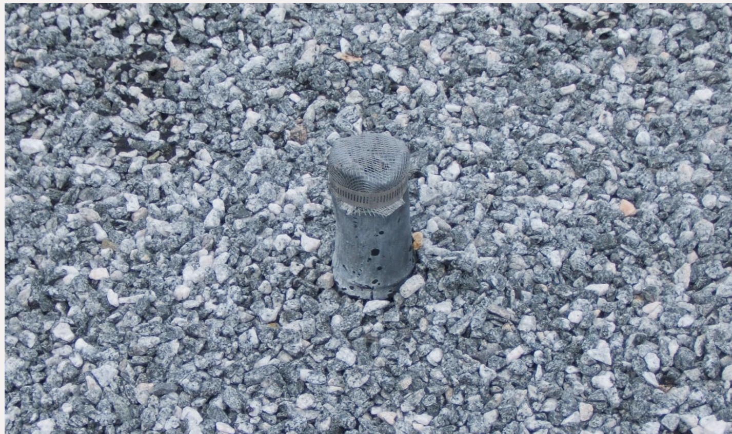
Figure 9: Vent stacks are normally 3" or 4" in diameter and stand 6" to 18" above the roof, depending on the location of the structure. In the northern climates with snow, the vent will stand higher.
