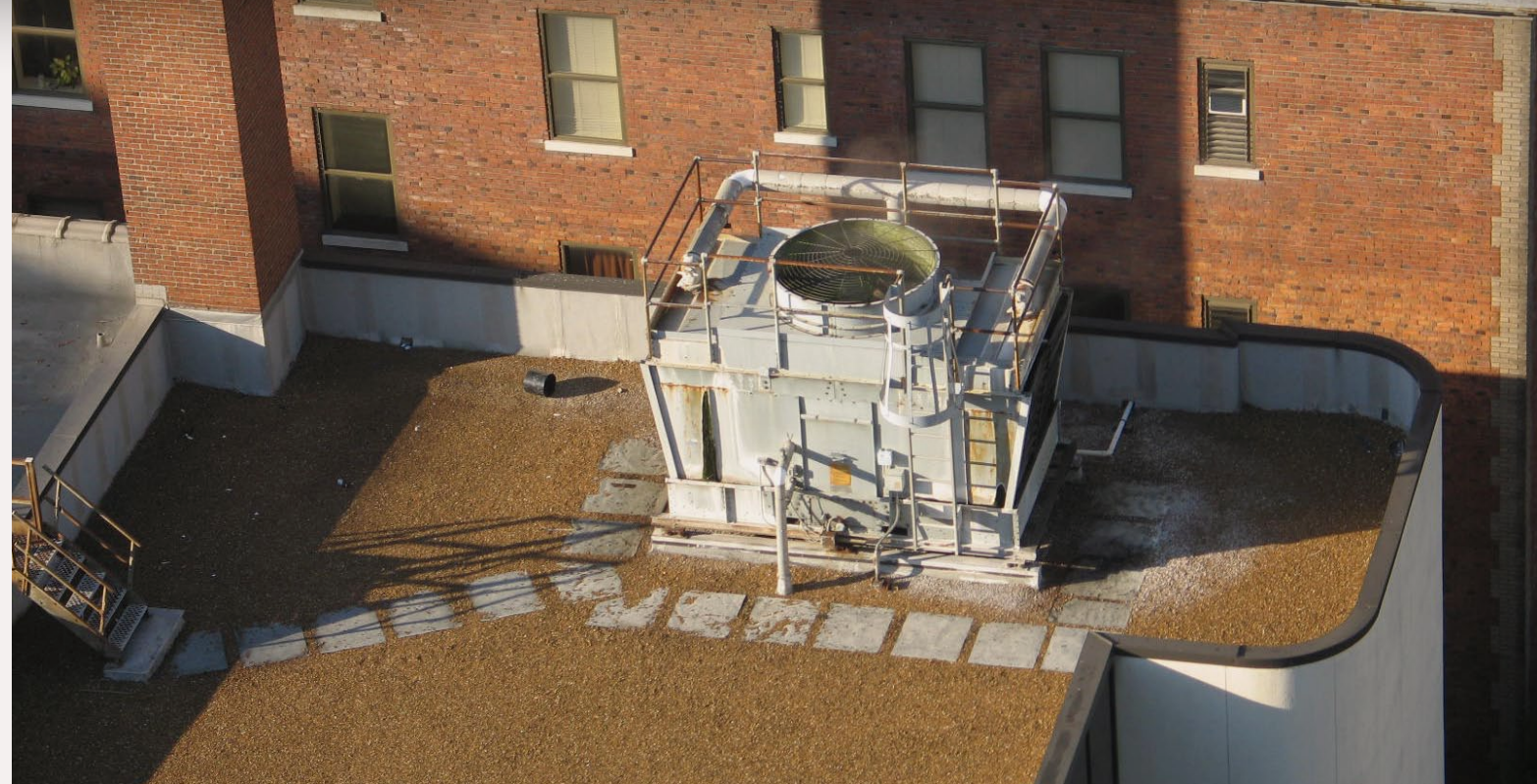
Figure 25: This a picture of a cooling tower. Piping coming out of the front goes to the chiller located in the building. Electrical disconnect switches are for the fan. The walkway pads protect the roof and the walkway stairs make it easy to access the unit for servicing.
