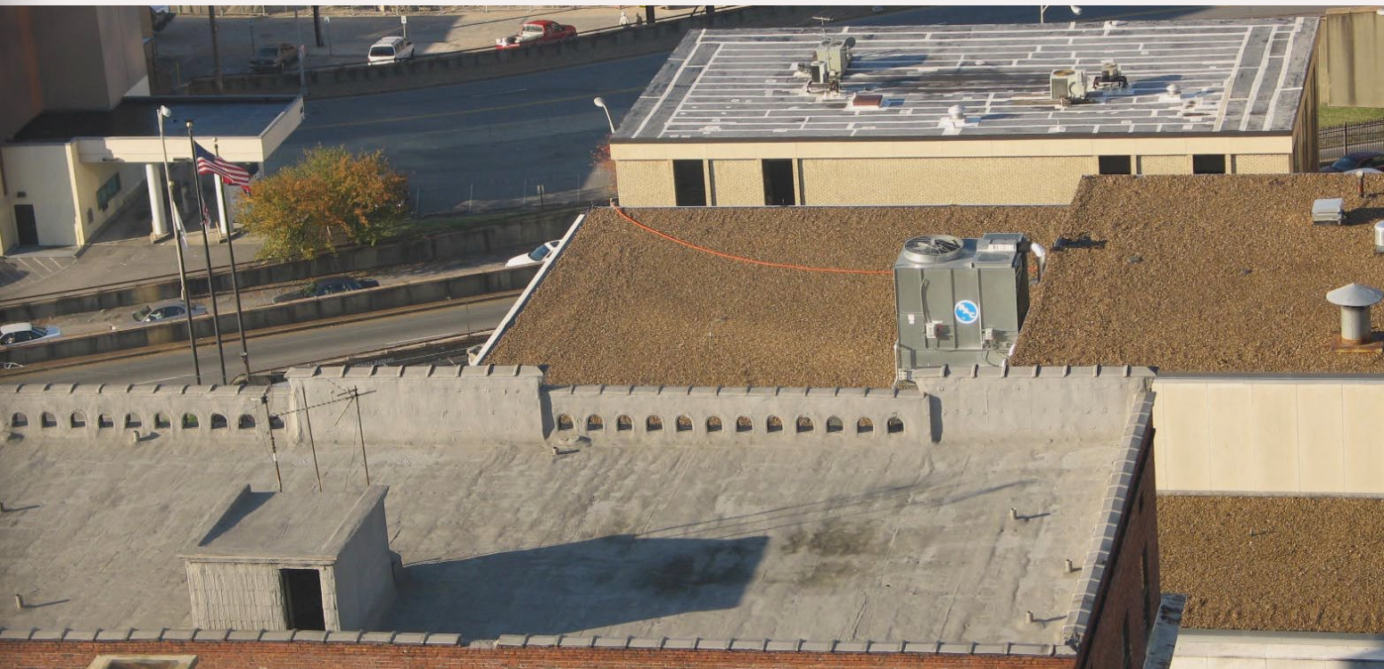
Figure 5: Here's a combination of different roof types from front to back: roll-down and tar-and-gravel. On the front building, notice the antenna on the roof access and the tile caps on the roof edge. A new cooling tower has been added to the second building's roof. On the rear building, repairs have been made to the roof.
