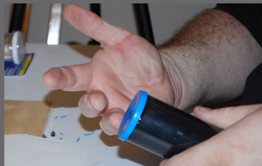
Figure 1.20: Firm downward pressure and a small twisting motion are all it took to firmly seat the cap in place, flush against the end of the pipe.
