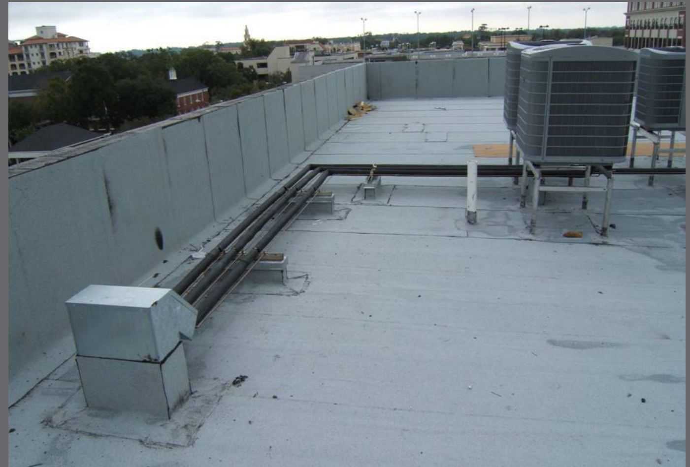
Figure 49: Typical installations showing the "dog house" where the piping comes out of the roof and goes on roof supports to the condensing units.
