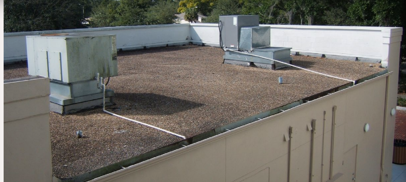
Figure 17: These are typical roof-top air conditioning units or furnaces. Note the drains from the units going to the roof gutter. Also notice the vent stacks for the sanitary system. The roof is tar-and-gravel having a turned-up membrane with flashing attached to the wall.
