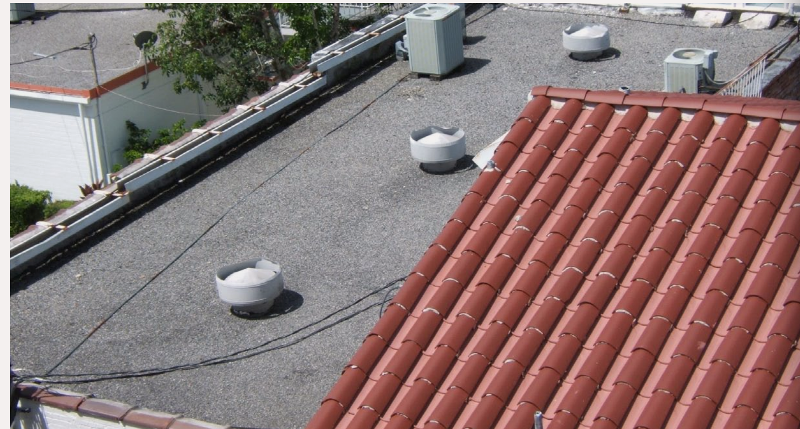
Figure 10: These are typical roof ventilators for a commercial flat roof. They let the heat escape from the attic. Notice the roof heights and types of roofing, and even the tree growing between buildings. Modeling these details from photos will enhance the scenes on your model railroad.
