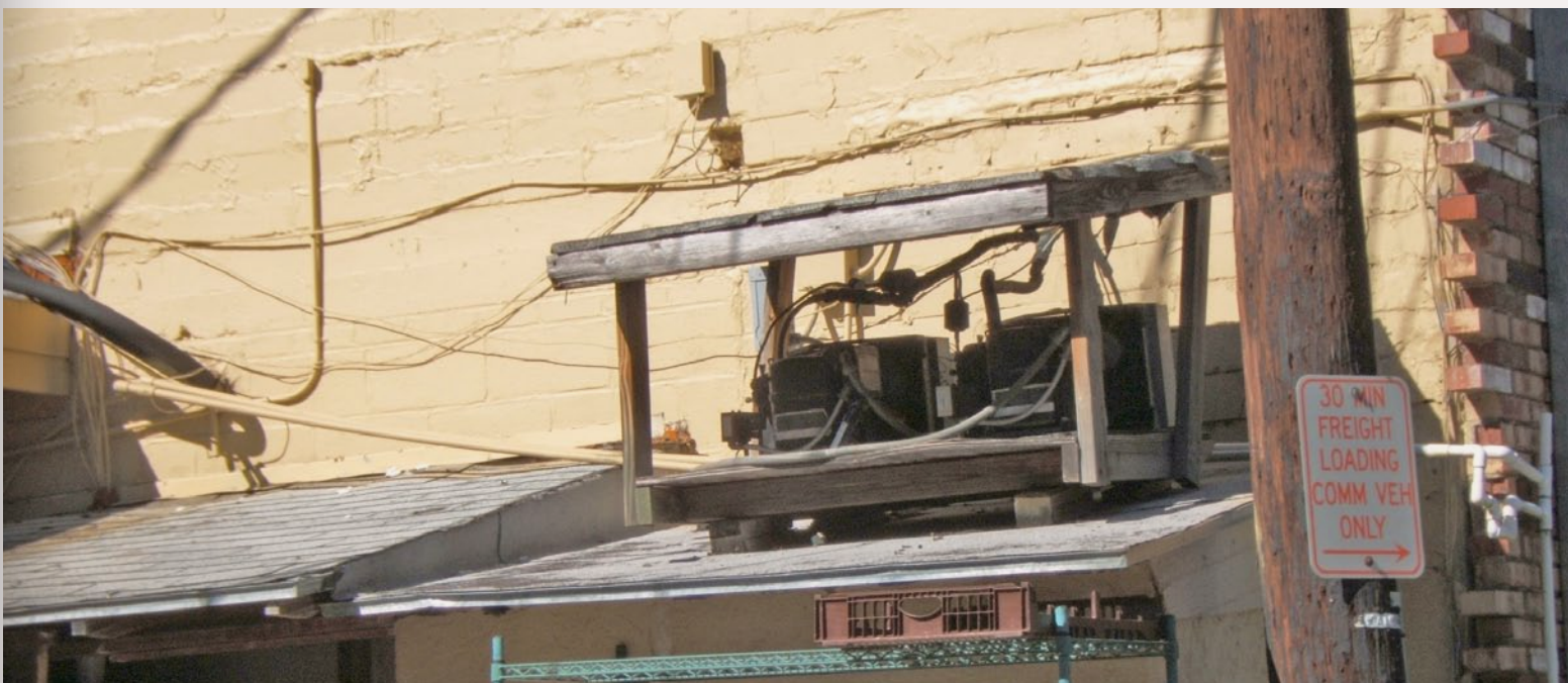
Figure 18: Here is a refrigeration unit that has a thrown-together look to it. This picture is the basis for a restaurant refrigeration unit on my layout. Things like this give character to the roof details and are easy to make.
