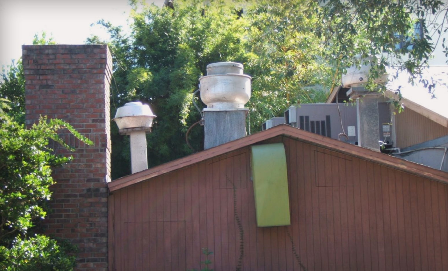
Figure 20: Multiple grease exhaust fans on the roof, with a makeup air duct on the wall (green ductwork).
