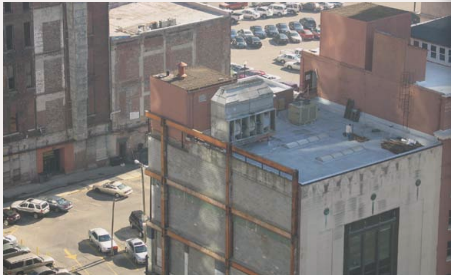
Figure 26: Another style of cooling tower.
