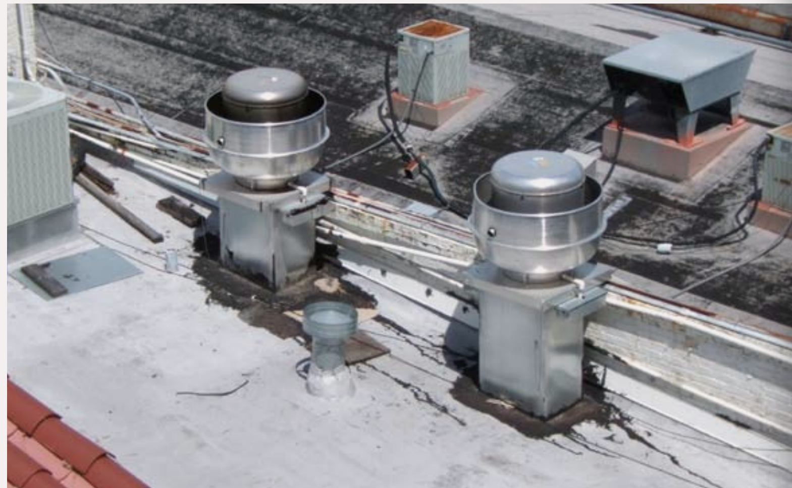
Figure 19: These two cooking-pot like vents are up blast grease exhaust fans. These units tilt so they can be cleaned. They stand 40" from the roof surface to the top of the fan.
