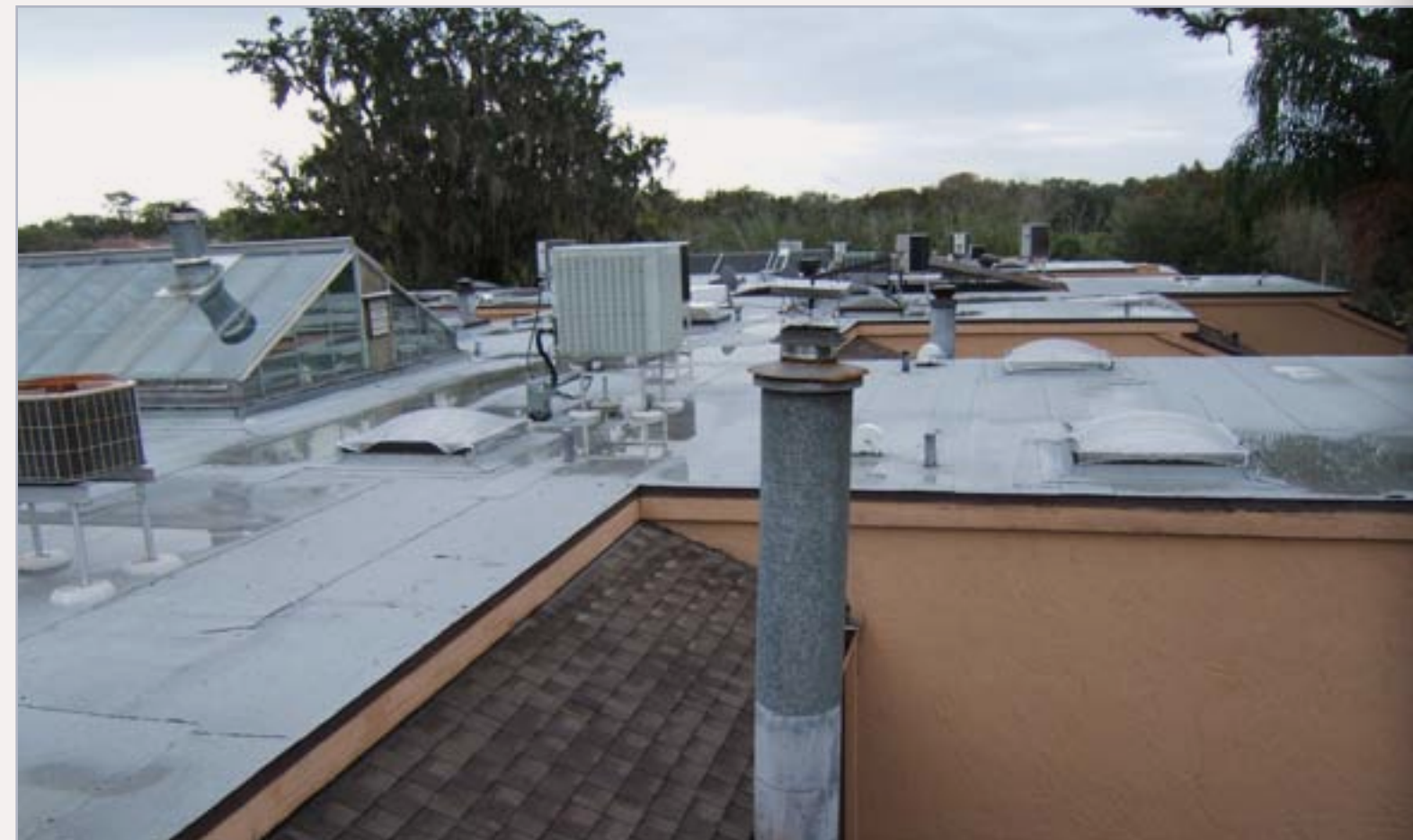
Figure 23: This house roof has a greenhouse. That big gray pipe in the foreground is a vent from a wood-burning fireplace.
