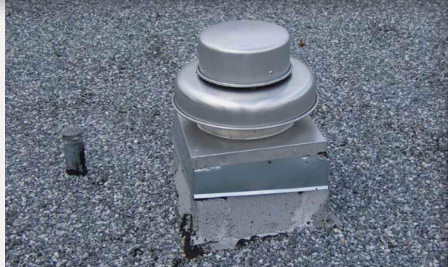
Figure 21: Restroom exhaust fan.
