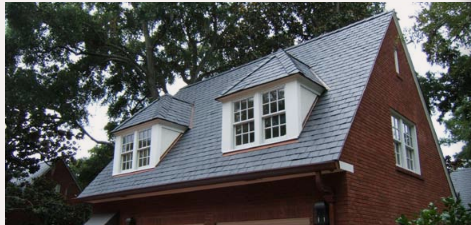
Figure 6: You won't find a slate roof used much in modern construction due to cost. A slate roof will last 50 years or more – this brand-new slate roof was installed to match the original house.
