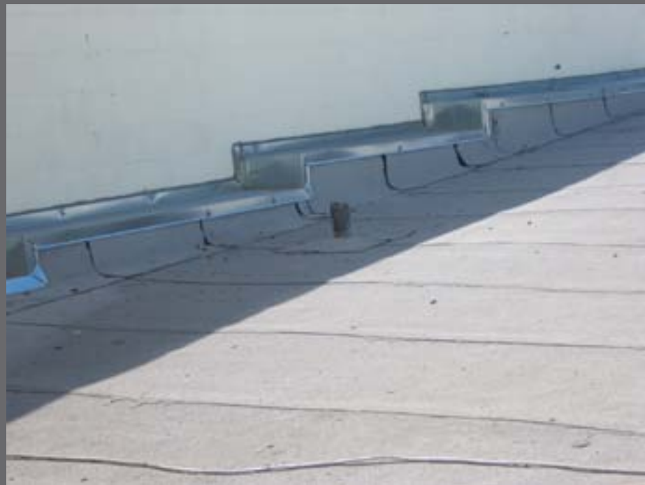
Figure 47: Prototype picture showing step flashing installed. Notice that the tar from the built up roof is not neat.
