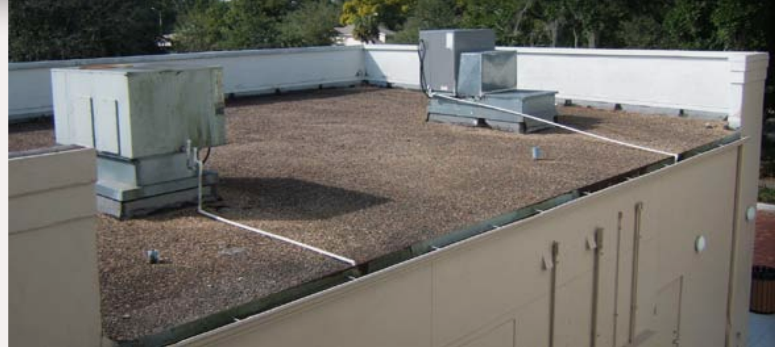
Figure 17: These are typical roof-top air conditioning units or furnaces. Note the drains from the units going to the roof gutter. Also notice the vent stacks for the sanitary system. The roof is tar-and-gravel having a turned-up membrane with flashing attached to the wall.
