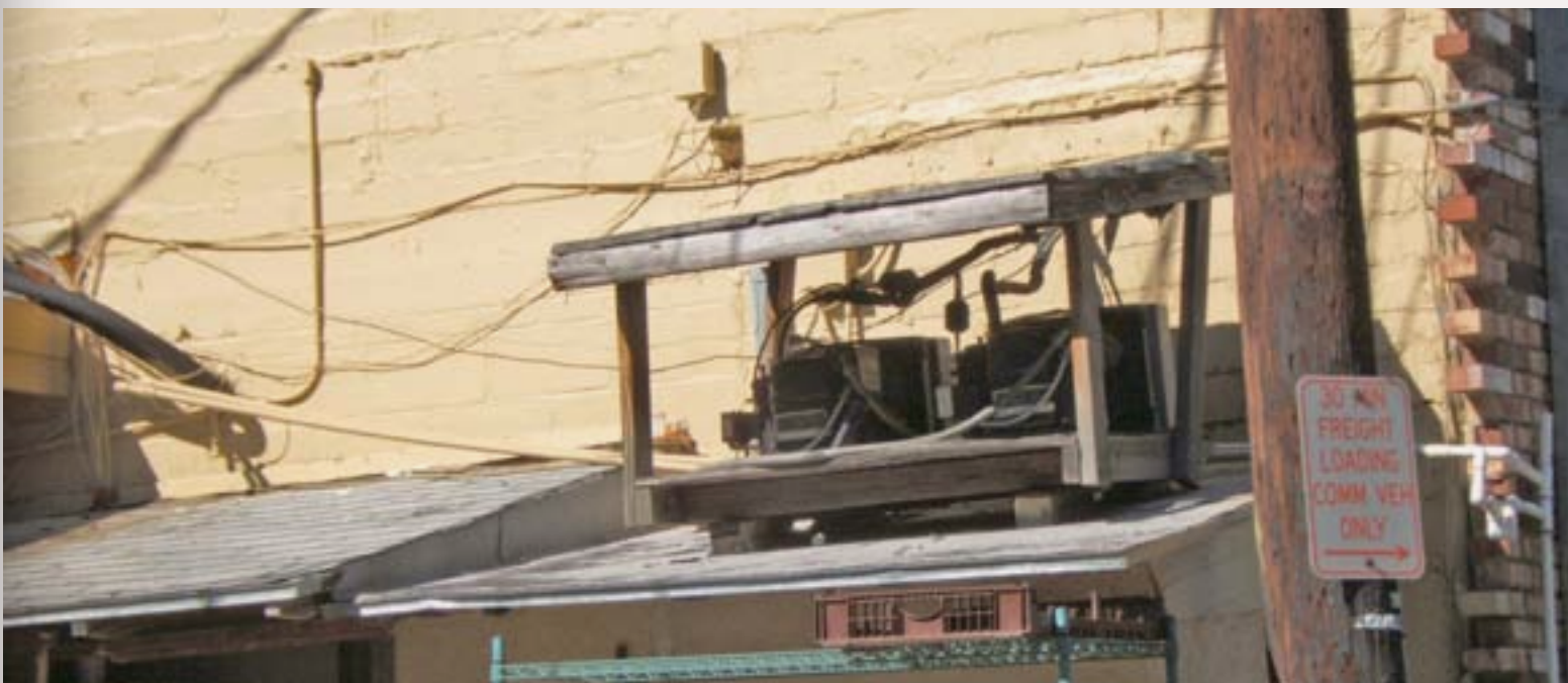
Figure 18: Here is a refrigeration unit that has a thrown-together look to it. This picture is the basis for a restaurant refrigeration unit on my layout. Things like this give character to the roof details and are easy to make.
