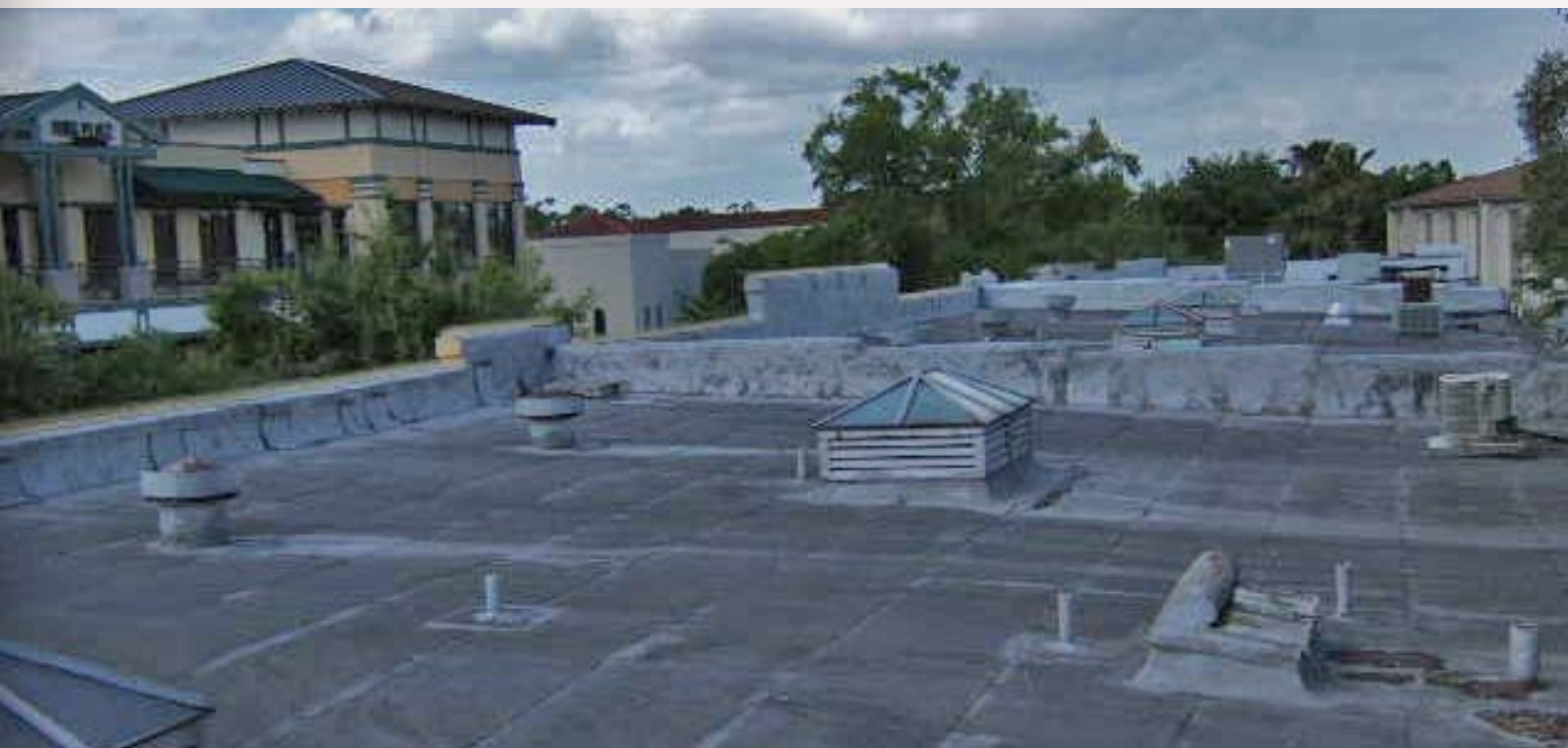
Figure 22: Typical roof details as seen from 1920 through today. This roof has old-style skylights installed (Campbell Scale Models and Grandt Line make this style of skylights). This roof also has old-style roof ventilators with very noticeable weathered streaking. The galvanizing on the smaller pipe ventilators keeps them from exhibiting such strong streaking.
