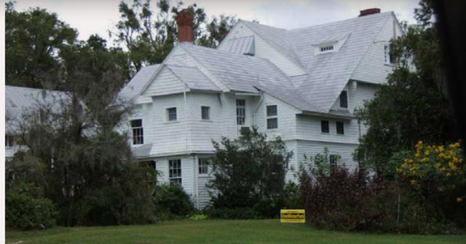
Figure 8: This house has a metal-stamped roof . Normally you will see the corrugated type or the standing-seam type. This style was made to look like shingles, but being metal gives better fire protection than shingles.
