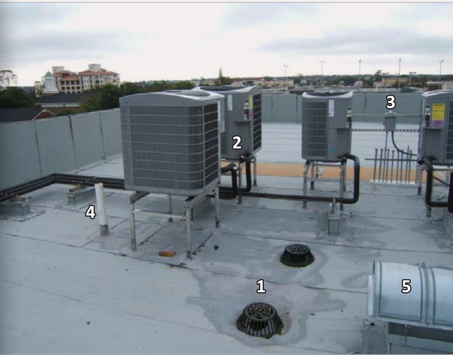
Figure 24: This a modern installation on a roof showing :
