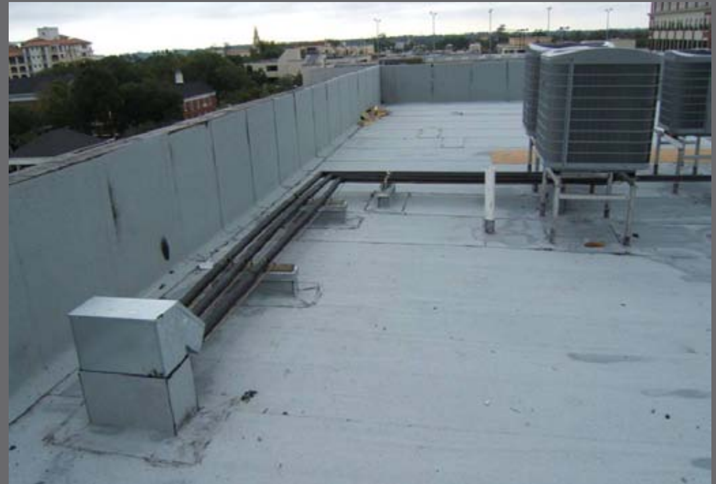
Figure 49: Typical installations showing the "dog house" where the piping comes out of the roof and goes on roof supports to the condensing units.
