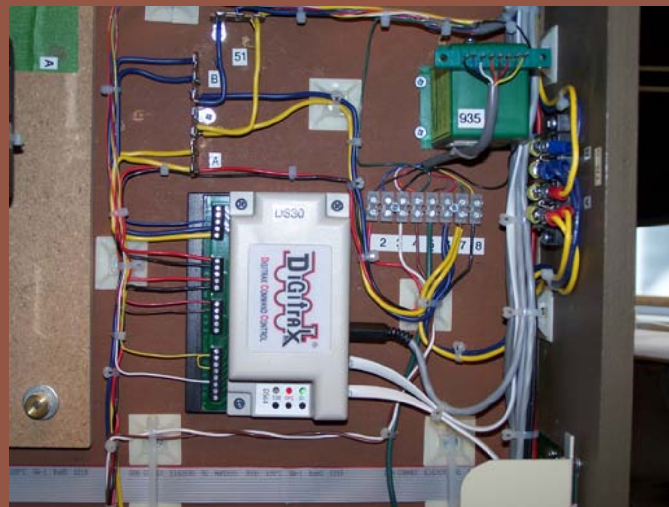
Figure 22: All three Tortoises hooked up to the DS64. I'm not particularly proud of the routing of the wires here. I'll do better next time!
