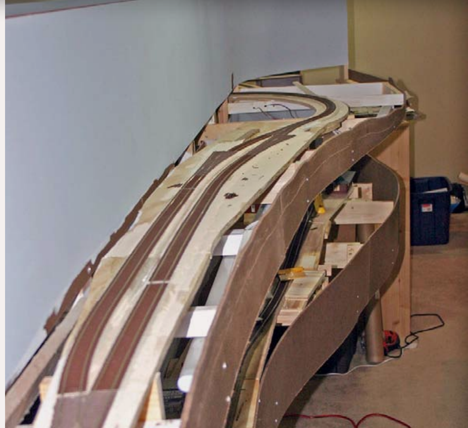
FIGURE 7: The siding at Milton was really not long enough. One evening session of about an hour was all it took to remove the track, add new subroadbed and roadbed, and replace the track. The last five minutes were spent putting the shop vac to use!
