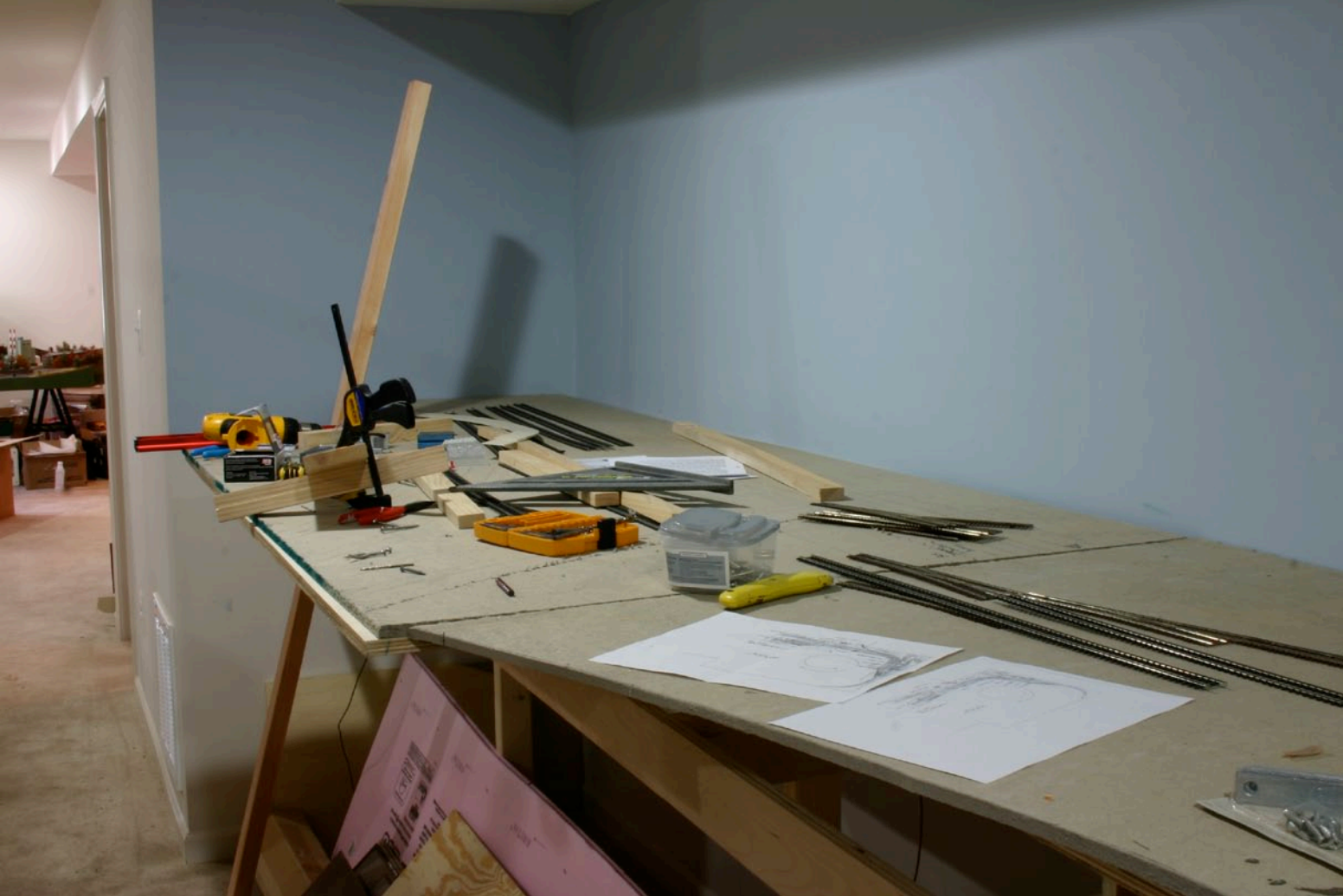
FIGURE 2: This photo shows the pier area in the early benchwork stages. The narrow aisle to the left of the short wall is visible. It was impractical to penetrate that short wall because the HVAC is on the other side.
