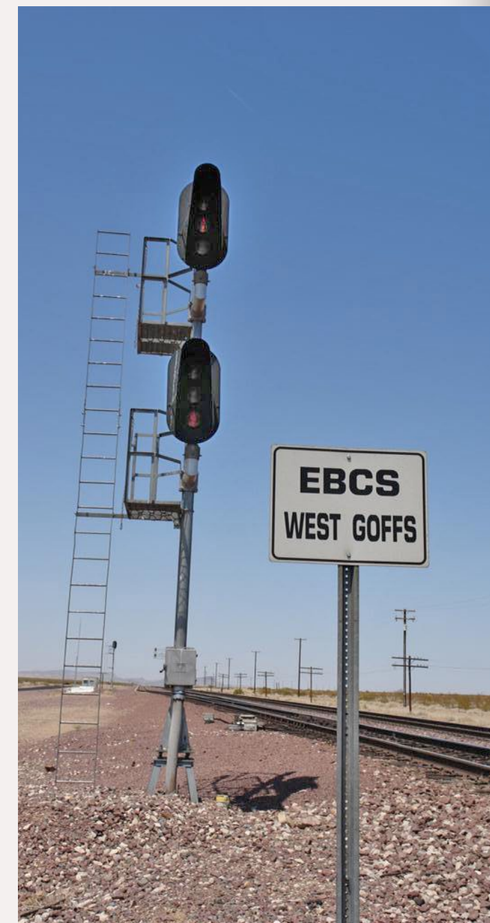
Figure 7. Eastbound signal mast.
