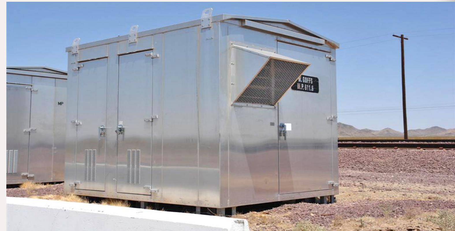
Figure 2. West and south sides of the generator cabinet.
