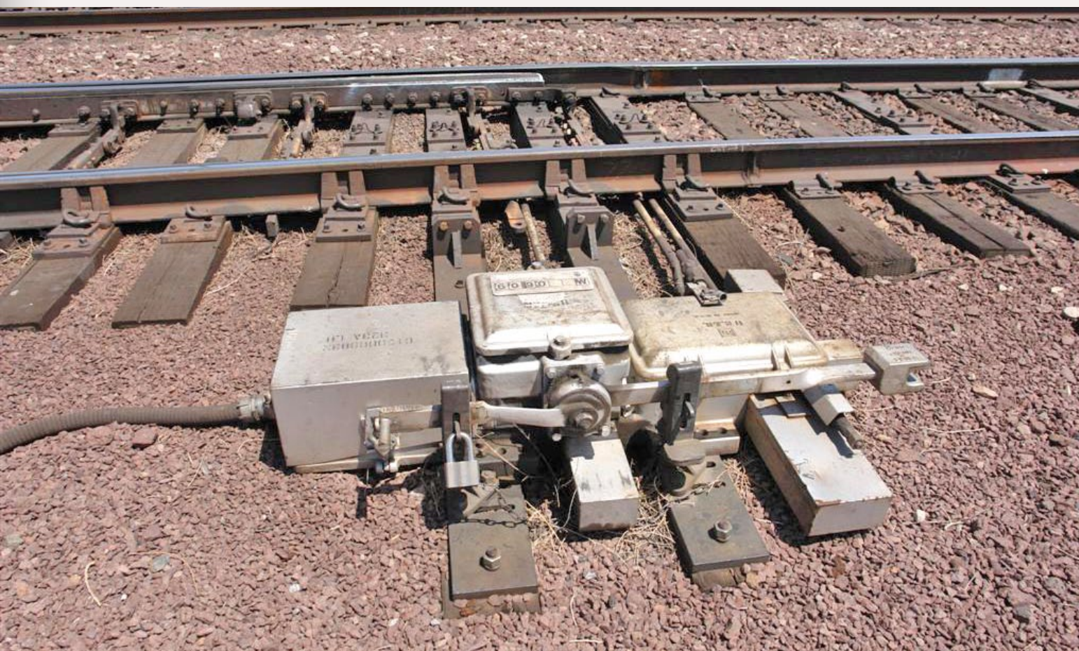
Figure 9. West Goffs remote switch.
