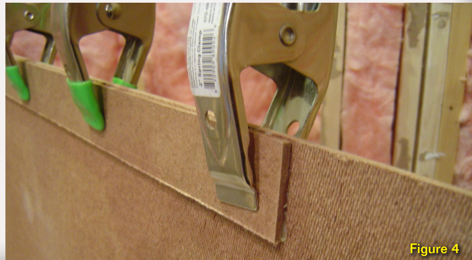
Figure 4: Since the hardboard butts up to \frac{1}{2} " drywall, I laminated a 1\frac{1}{2} " wide strip of \frac{3}{16} " thick hardboard to the unfinished (back) long edge of the 4' x 8' sheet of hardboard using white glue. Drywall that is \frac{1}{2} " thick tapers to \frac{3}{8} " on its long edge. By doubling the thickness of the hardboard with the additional strip, it becomes \frac{3}{8} " thick – the same thickness as the edge of the drywall.
