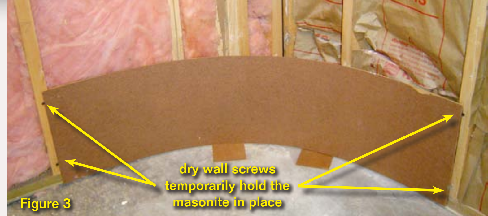
Figure 3: The first thing that I did was test-fit a piece of 2' high by 4' long by \frac{3}{16} " thick hardboard in the corner using some drywall screws screwed into the studs (not through the hardboard) to hold it in place. The stud spacing, 28\frac{1}{2} " from the corner in both directions, allowed for an attractive curve with the hardboard fitting flat against the studs. If the stud spacing wasn't acceptable, I would have added intermediate studs.
