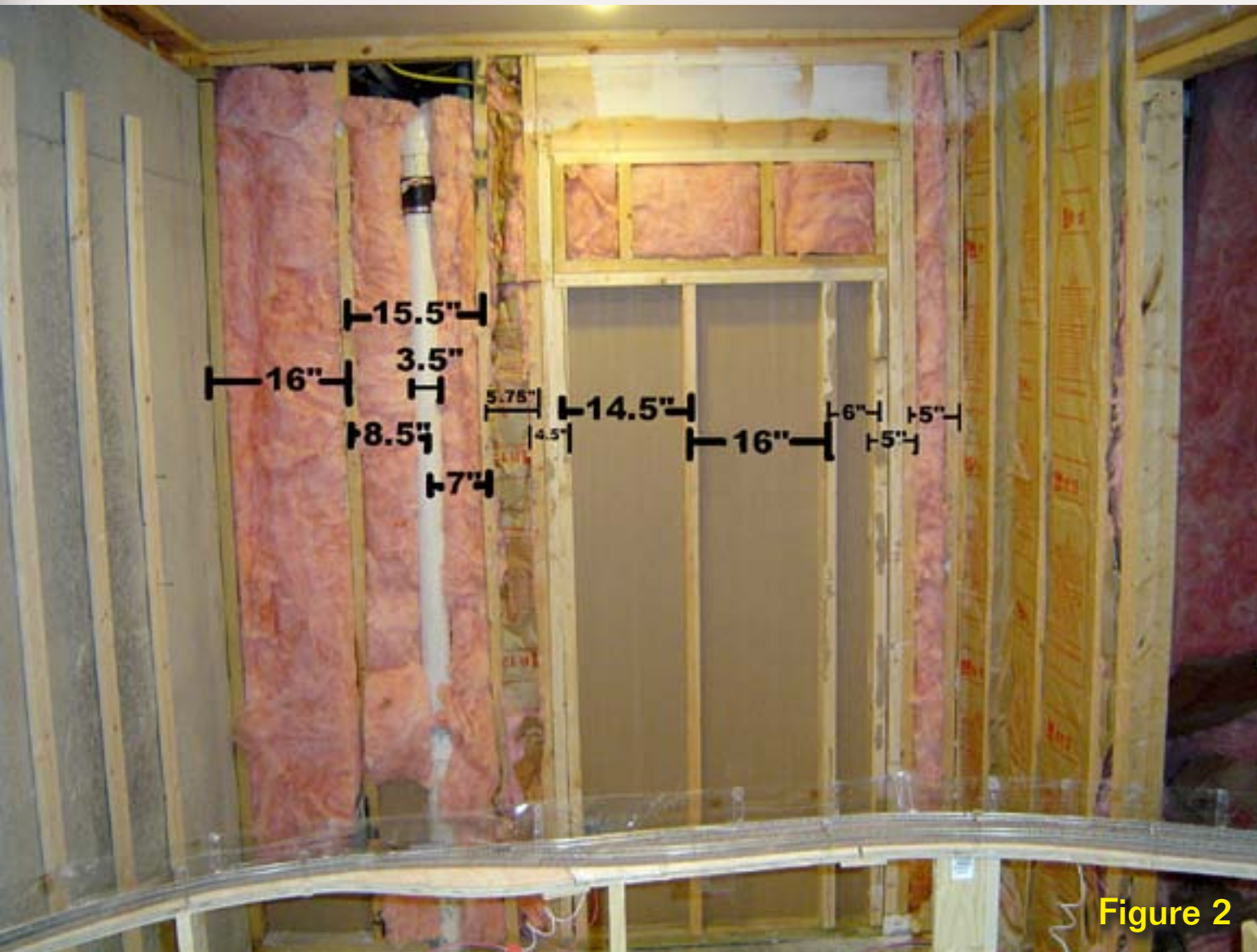
Figure 2: Here is the reclaimed 6 x 7 space looking from the existing train room. I've studded-in the old closet entrance in the back wall and will close up the entrance that already existed to the right.
