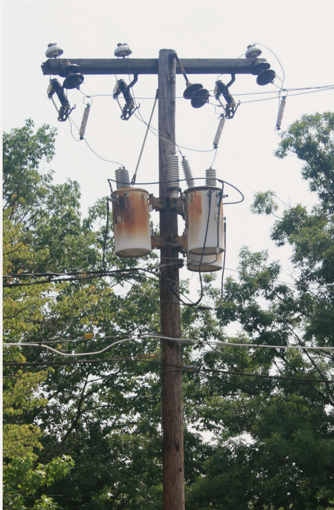
Figure 2: The rust on these transformers shows that the poles and wires have been in service for a while.
