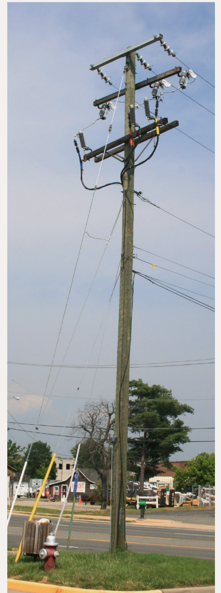
Figure 3: End poles often have one or more wires to stabilize them.
