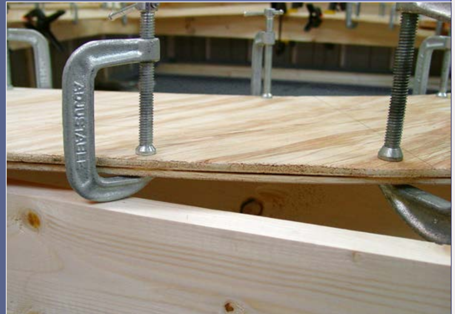
Figure 7a: We laminate two 1/4" layers of lauan plywood sub-roadbed together using carpenter's glue and clamps to get one 1/2" plywood sandwich. By staggering the joints in the layers, no joint splice plates are necessary.
