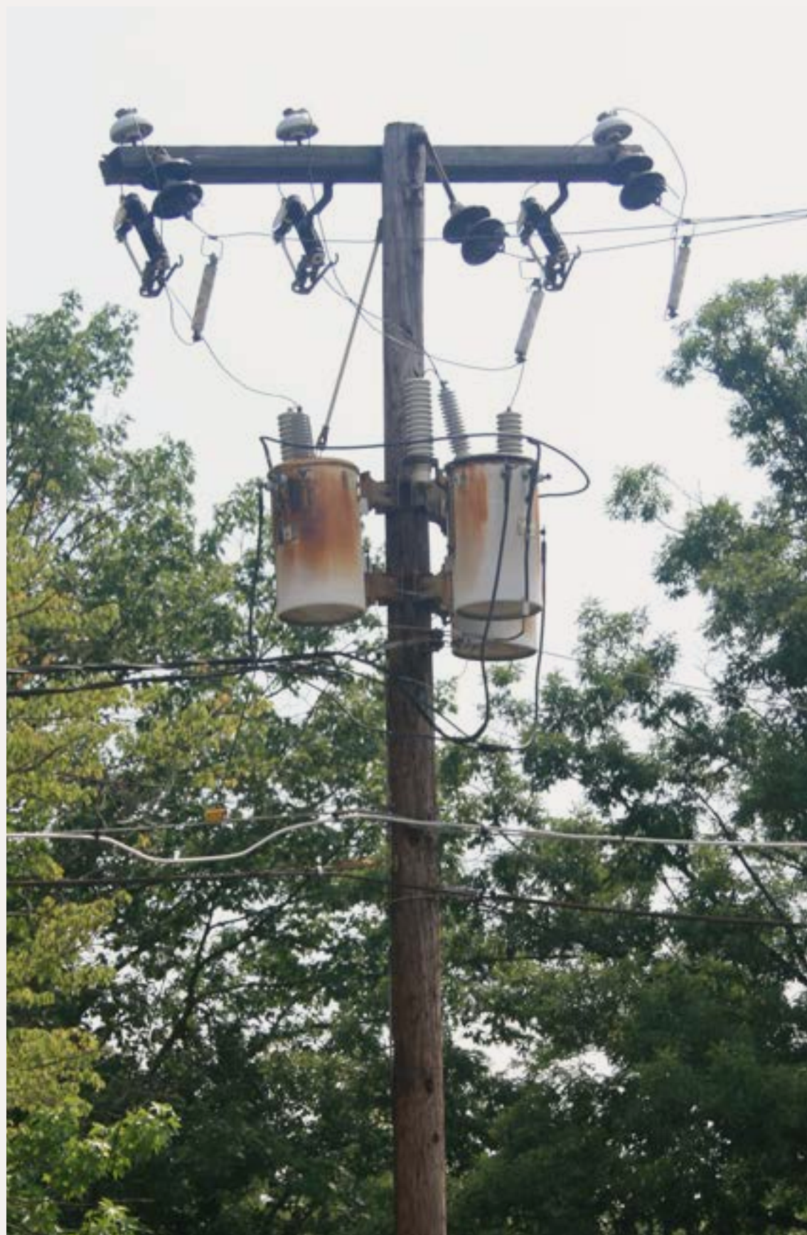
Figure 2: The rust on these transformers shows that the poles and wires have been in service for a while.
