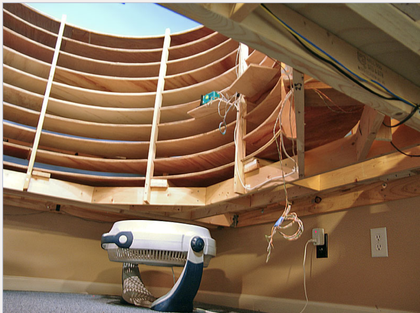
Figure 18: Fan in the center of the helix core for air movement.
