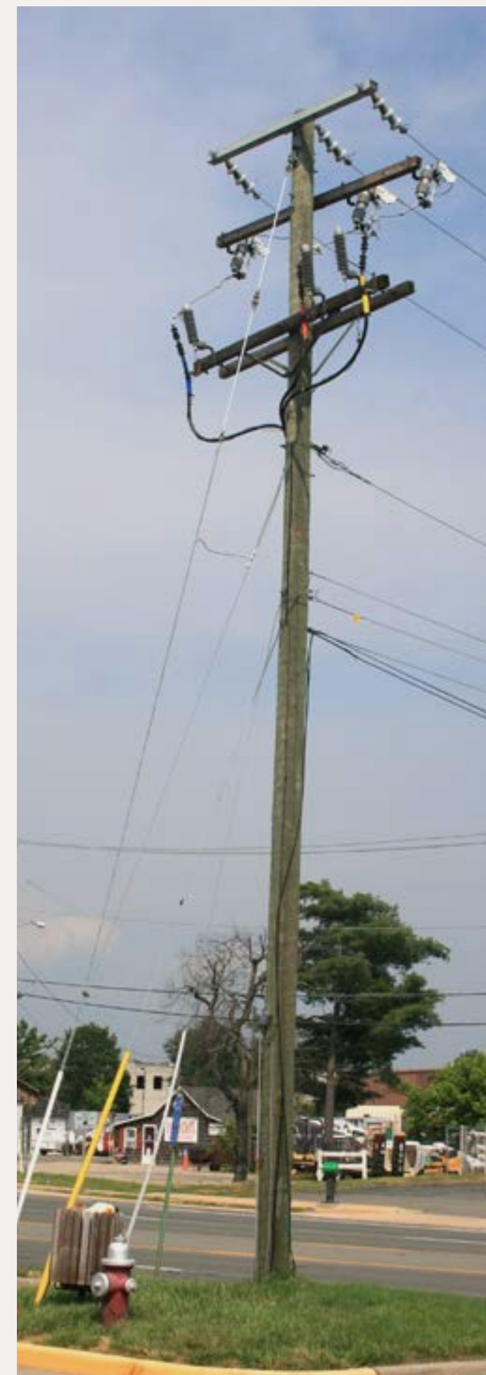
Figure 3: End poles often have one or more wires to stabilize them.
