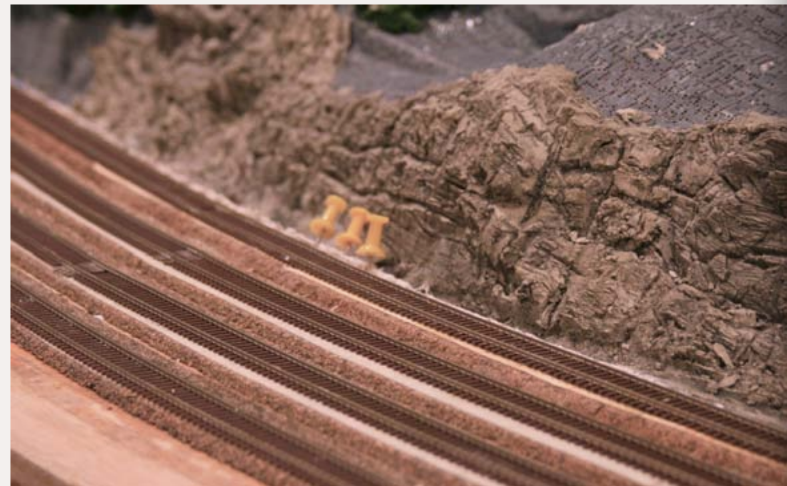
Figure 1: The first step in the ballasting process is to make sure trackwork is smooth, functional, and cleaned up from the construction process.
