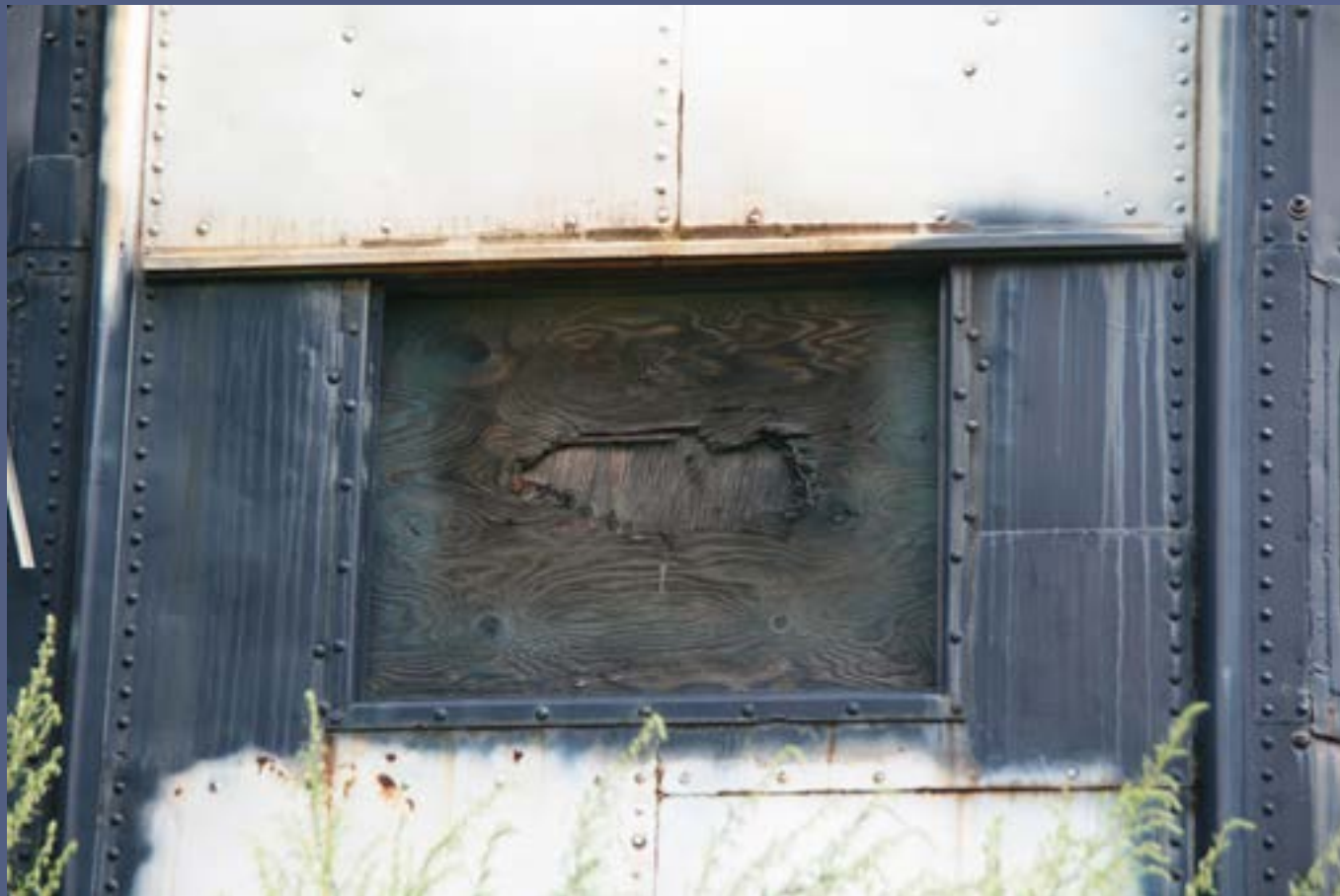
Figure 24: Plywood is often used to cover the windows of equipment that is in long-term storage. This removes a tempting target from vandals. The plywood covering the bay window of this caboose prevents weather from reaching the interior, causing further damage.
