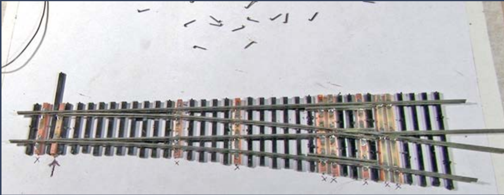
Figure 52: At this point turnout construction is basically finished, so I remove all the spikes from the PC ties. I leave the spikes holding the plastic ties since they need to remain in place until I'm ready to glue the turnout rails to them.
