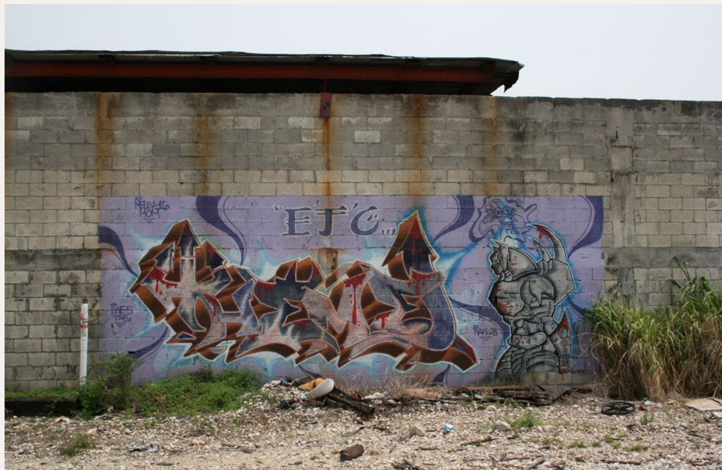
Figure 30: Graffiti 'art' on masonry wall.
