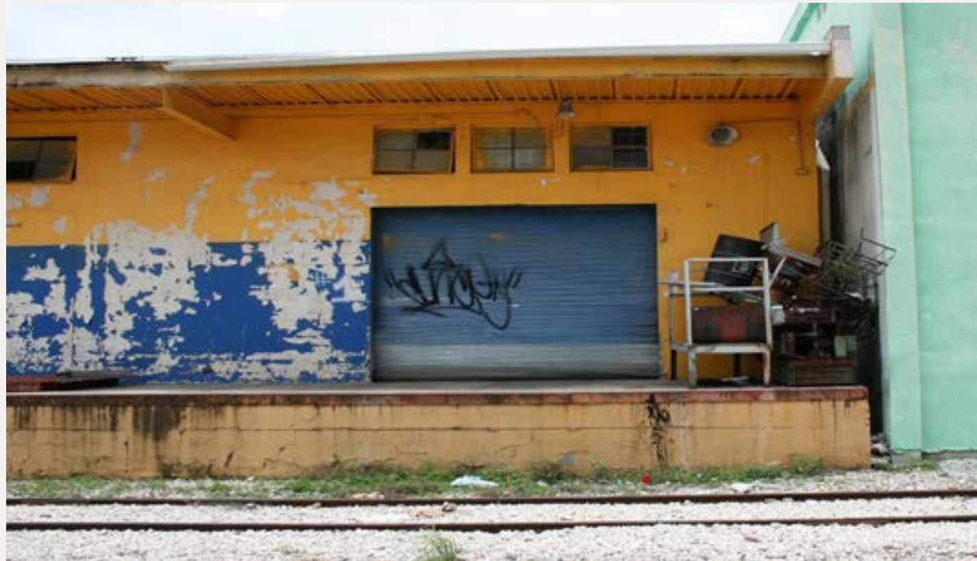
Figures 2: I can't imagine a project more difficult than trying to model this roll-up door with paint. The color combinations are very complex. The shallow relief between the slats is minute and typically not realistically produced with commercial door products. Time for the computer and printer.
