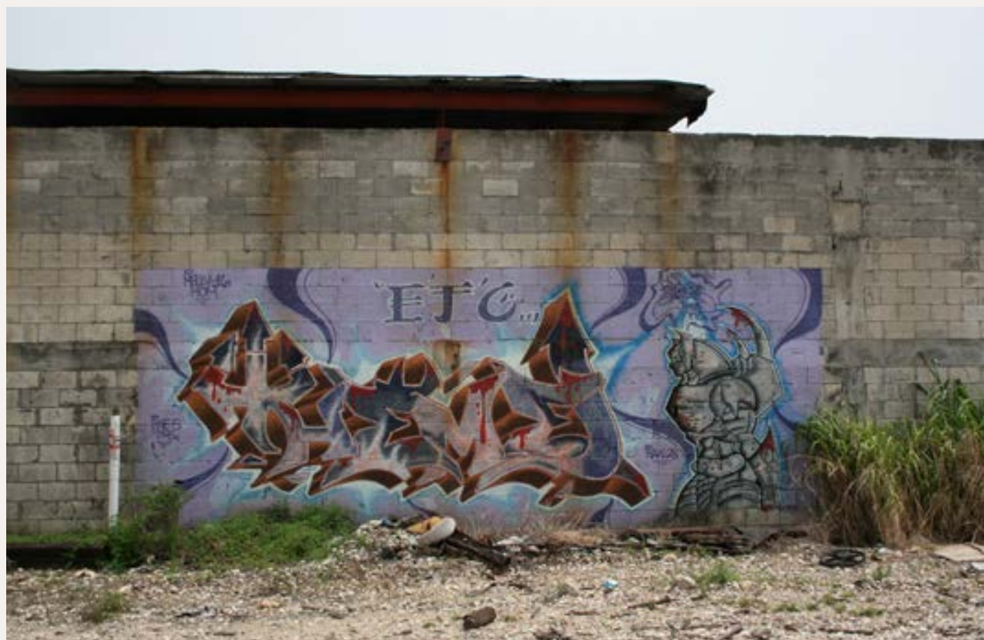
Figure 30: Graffiti 'art' on masonry wall.
