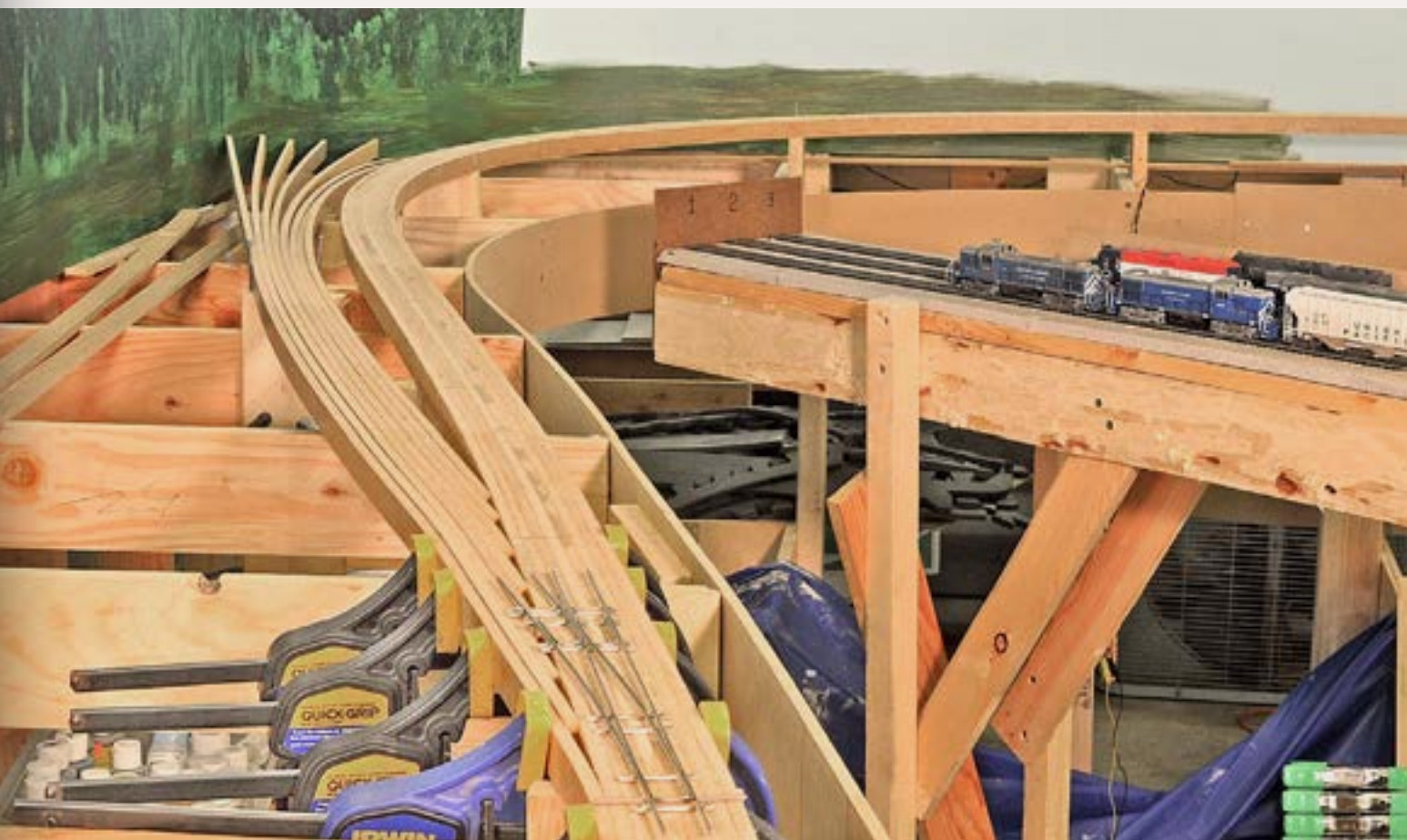
Figure 2: Smooth spline has to be laid out with care. This lay-up, with jagged edges abutting the main where the switch splits off to the left, was rejected in favor of attaching one long strip along the main and building the additional splines onto that.
