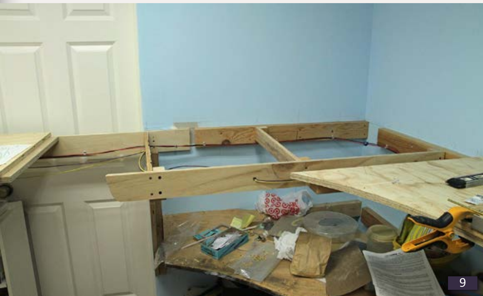
10. With the South Jackson roadbed set in place it's obvious where the turntable will get installed.
