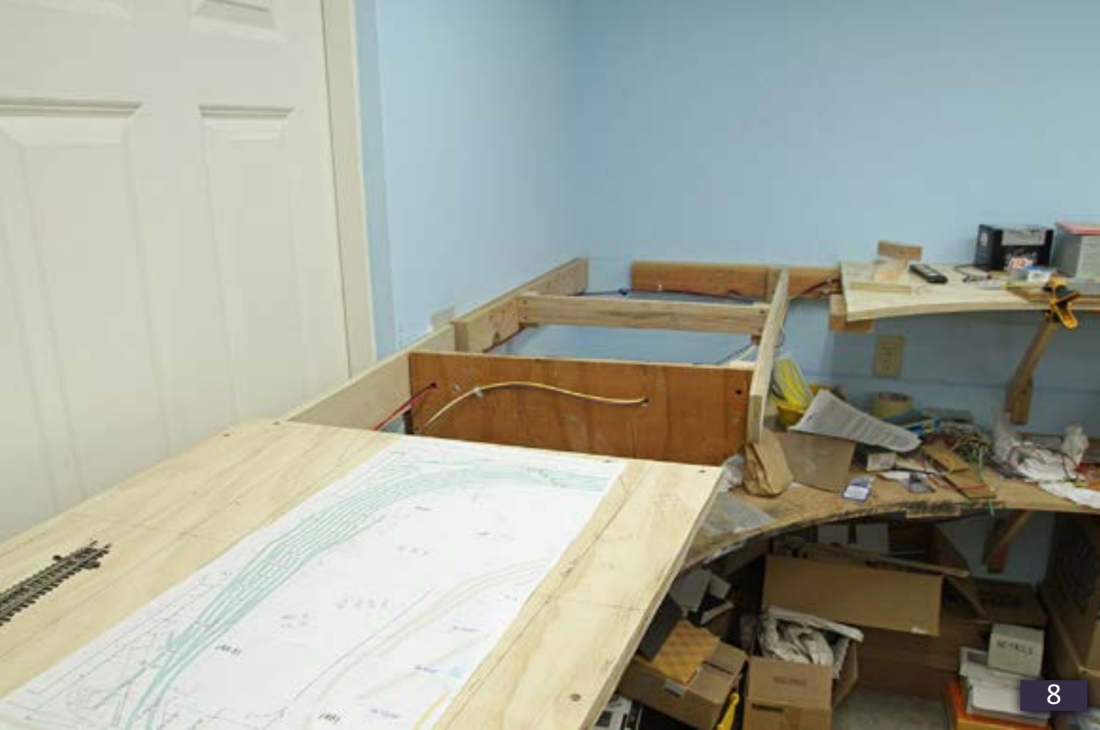
8, 9. South Jackson looking toward the turntable's corner. Most joists have been set in place and some wiring installed.
