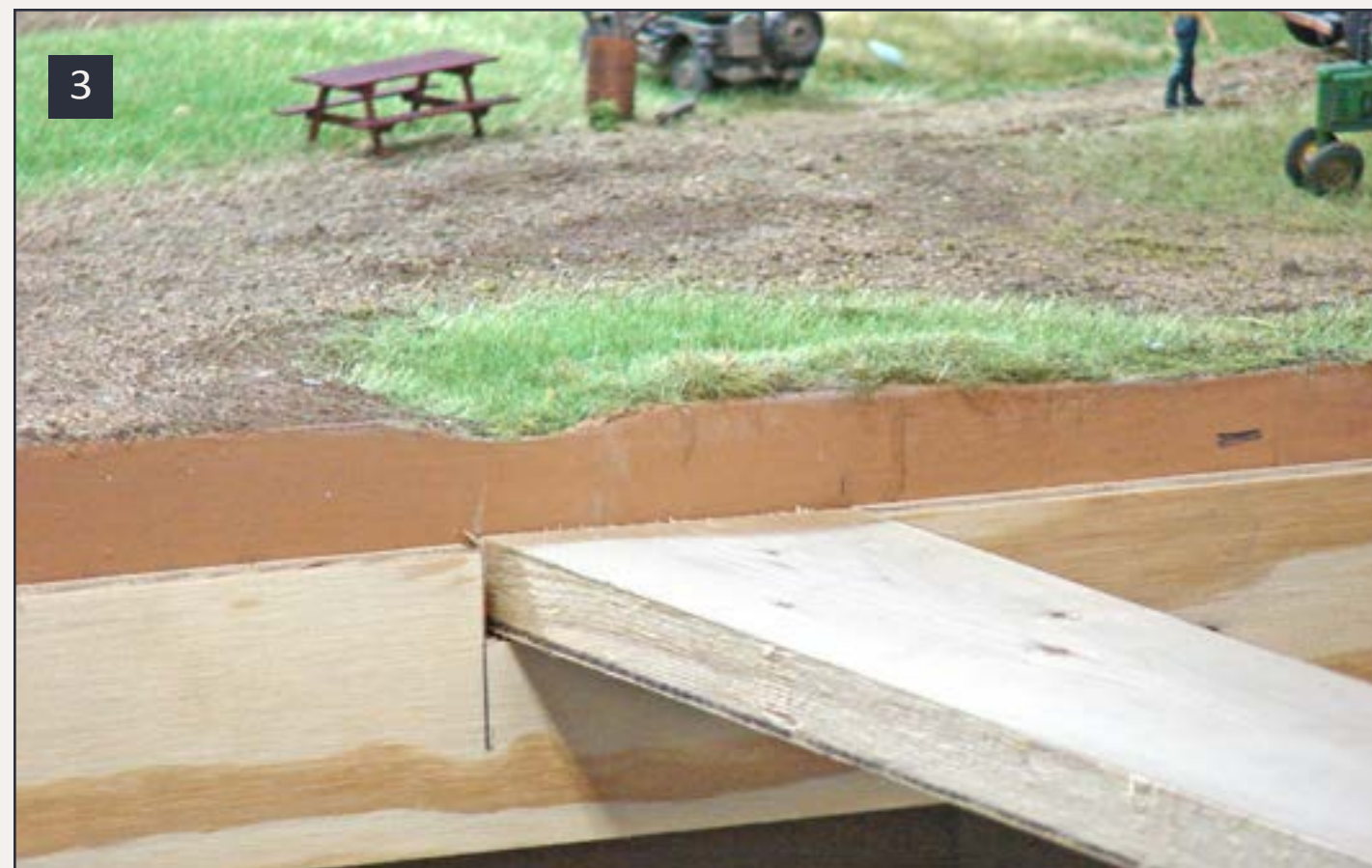
3: Adding notches into the plywood frame to hold the 1x4 support stringers.
