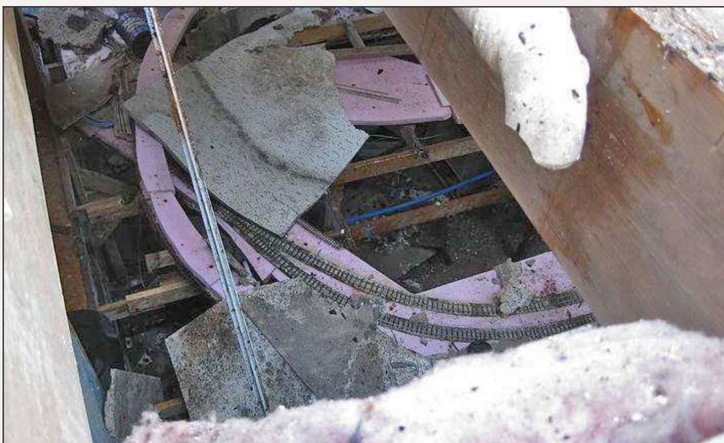
2: After the fire – a view of Peter’s layout from outside the house – photo courtesy of Peter Herron.
