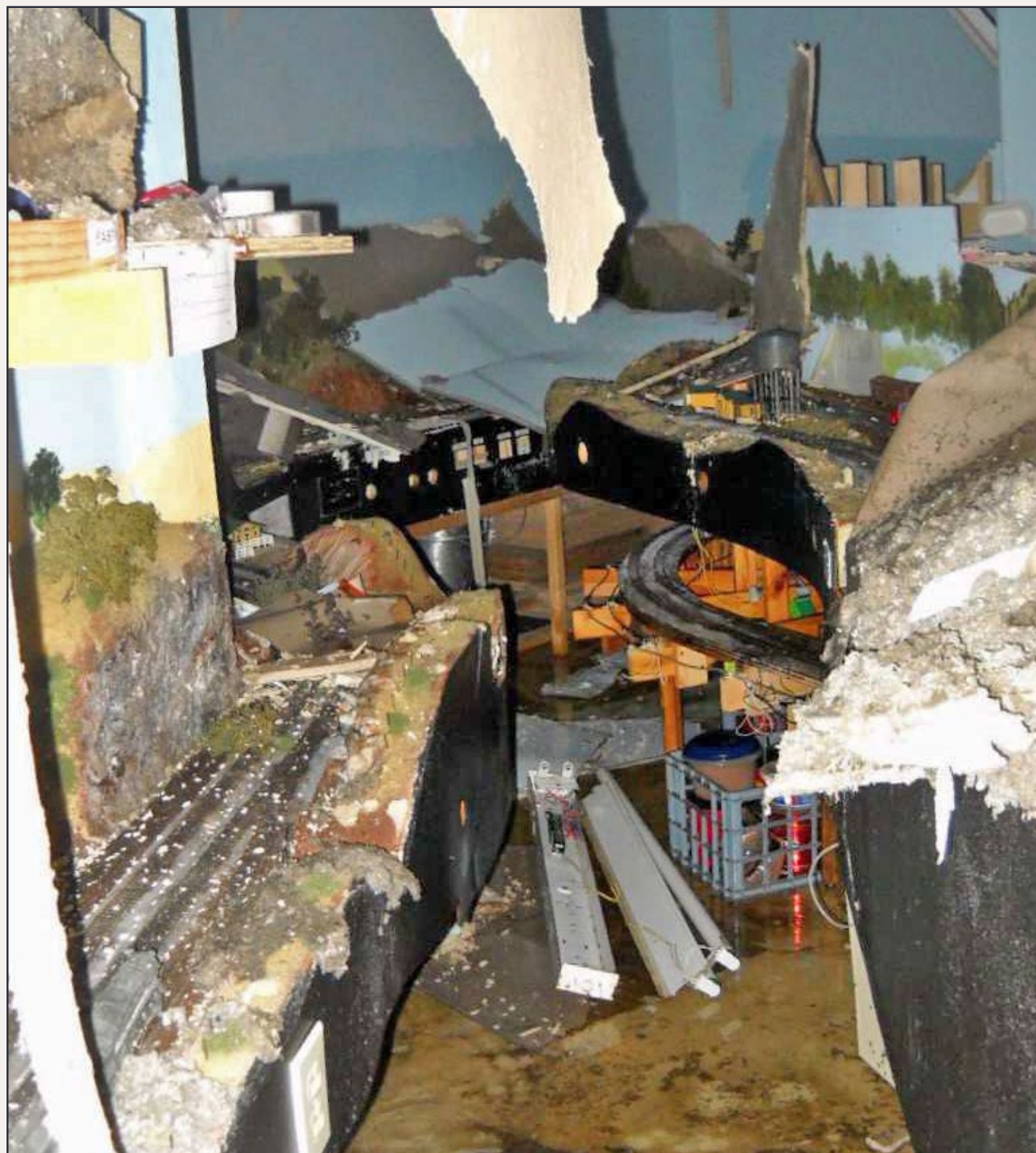
3: The water damage at Richard Newkirk's layout – photo courtesy Richard Newkirk.
