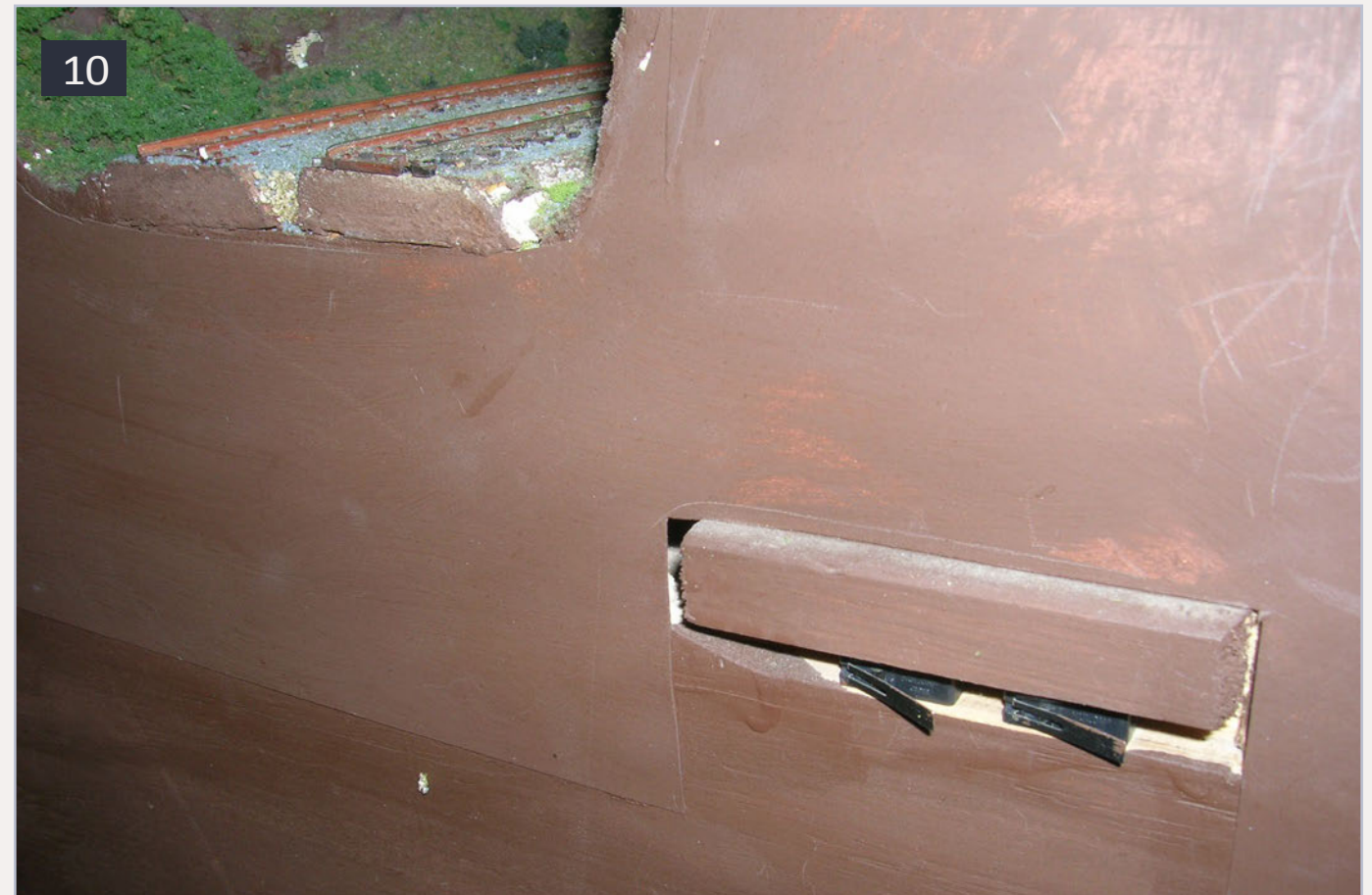
7. Detail of limit switches.
