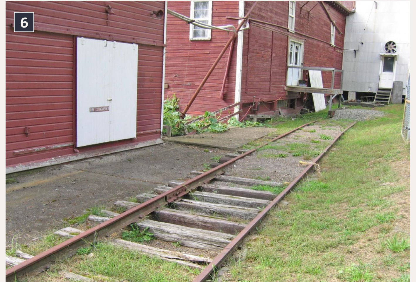
6: Here you can see the concrete that was part of the loading pit, now filled-in. It also looks like a truck dock has been built where rail cars once stood.
