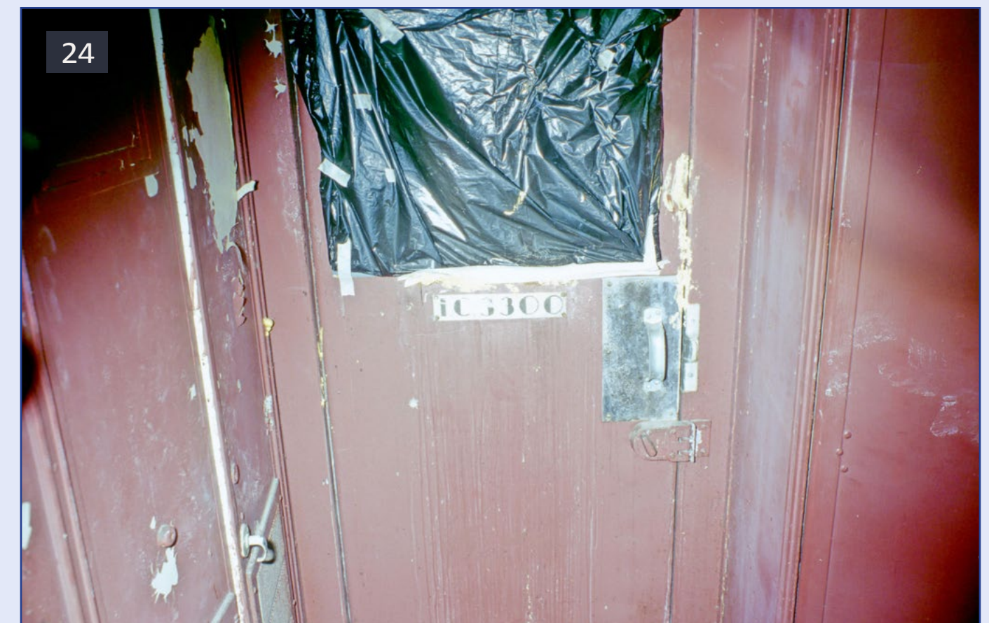
24: The I.D. plate still in place on the door.
