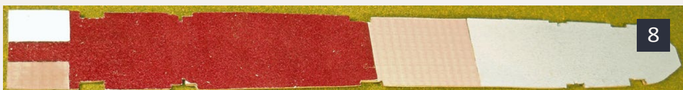
8: All of the flooring has been placed. The parquet tiles have a basket weave pattern that contrasts nicely with the carpet.
