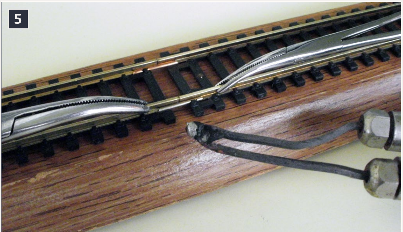
5. Clips on either side of a soldered rail joint draw heat away from the work and keep plastic ties from melting. Ronald D. Smith photo.
