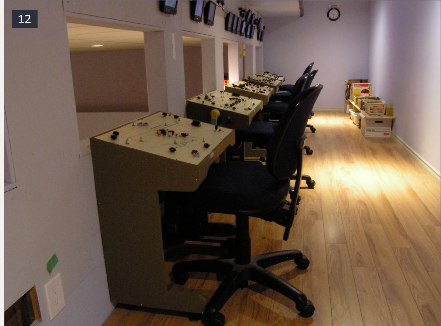
12. The finished control room. Each desk controls a section of the railway, as described in the text. Each monitor is connected to two cameras, which gives the operator of that area good top-down views of areas where there are uncoupling magnets, or hard-to-see switch locations.
