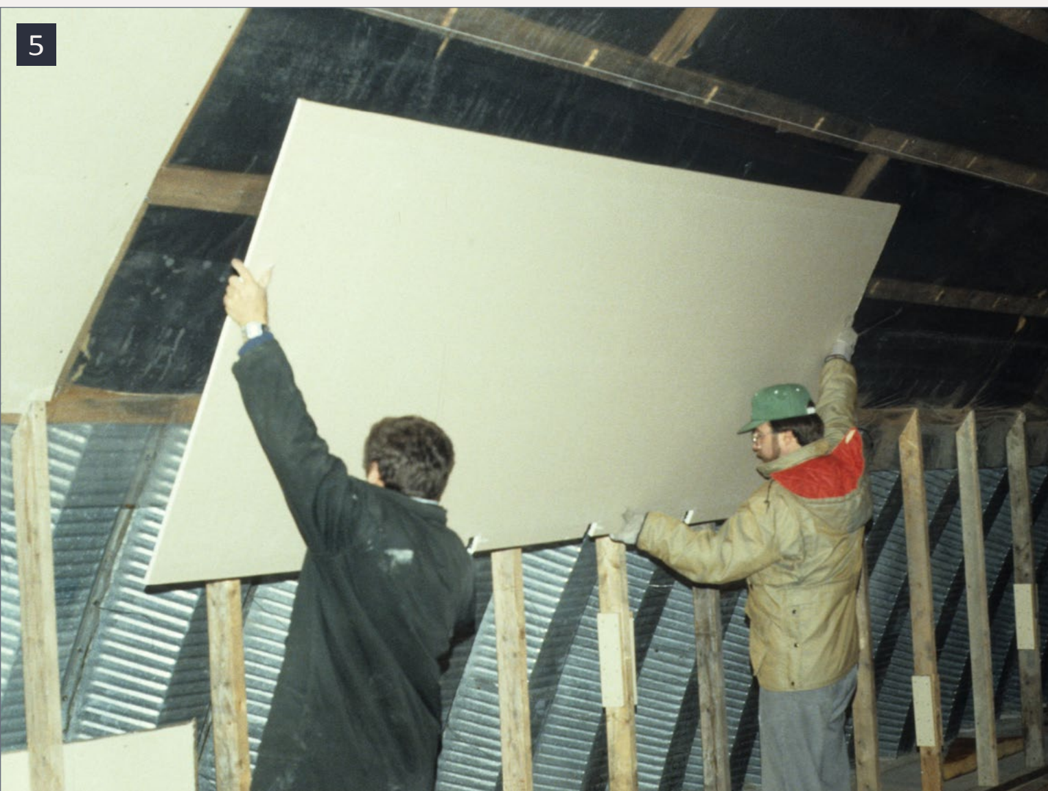
5. Adding sheets of drywall to the framing in the Quonset hut, November 1982.
